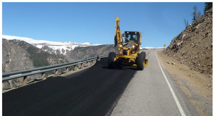
Paving on the Beartooth Highway in May 2026 (ahead of opening to seasonal traffic).
