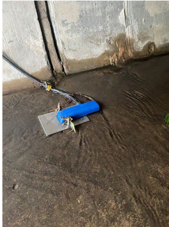
Figure 4-6. Example of Flow Sensor Installation
