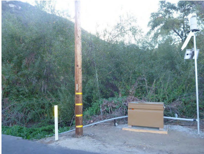
Figure 4-7. Example of Permanent Automated Sampler Enclosure
