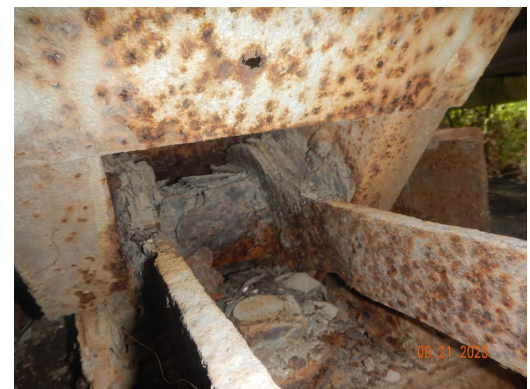
Photo 5: Eyebar section loss at L0' (South Truss)
