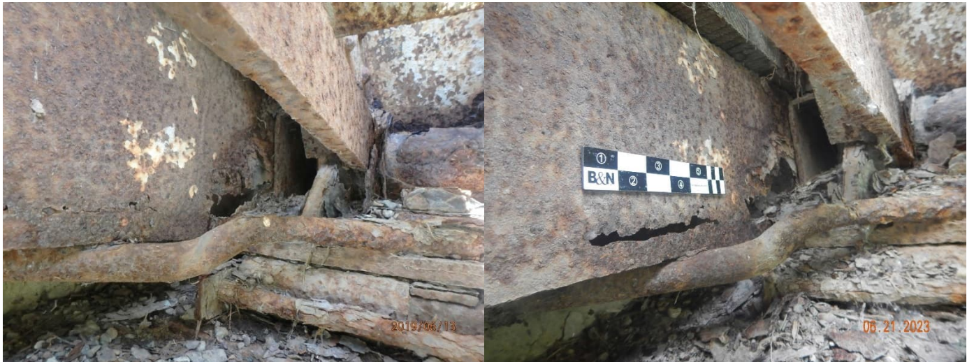
Photo 4: Progression of Section Loss in Stringer 8 web at Abutment 2 (2019 to 2023)
