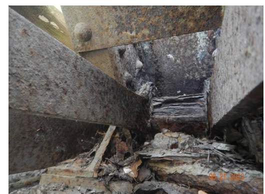
Photo 6: Severely corroded pin at L0 (South Truss)
