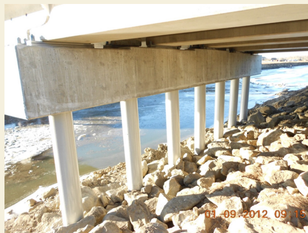
Figure 1: Typical MDT concrete-filled steel pile and concrete pile cap bridge substructure support system.
