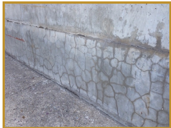
Figure 1: Typical ASR Crack Pattern
