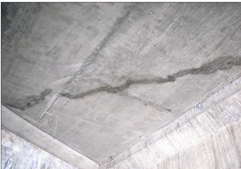
← Example image of full depth crack underside in the travel lane, east bound.
