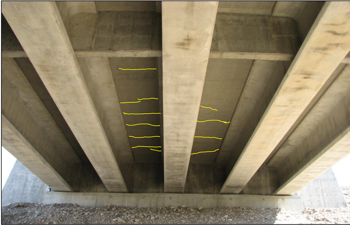
↑ West Bound Deck – East End: SD Placement ; a yellow line is superimposed to better delineate the crack.
