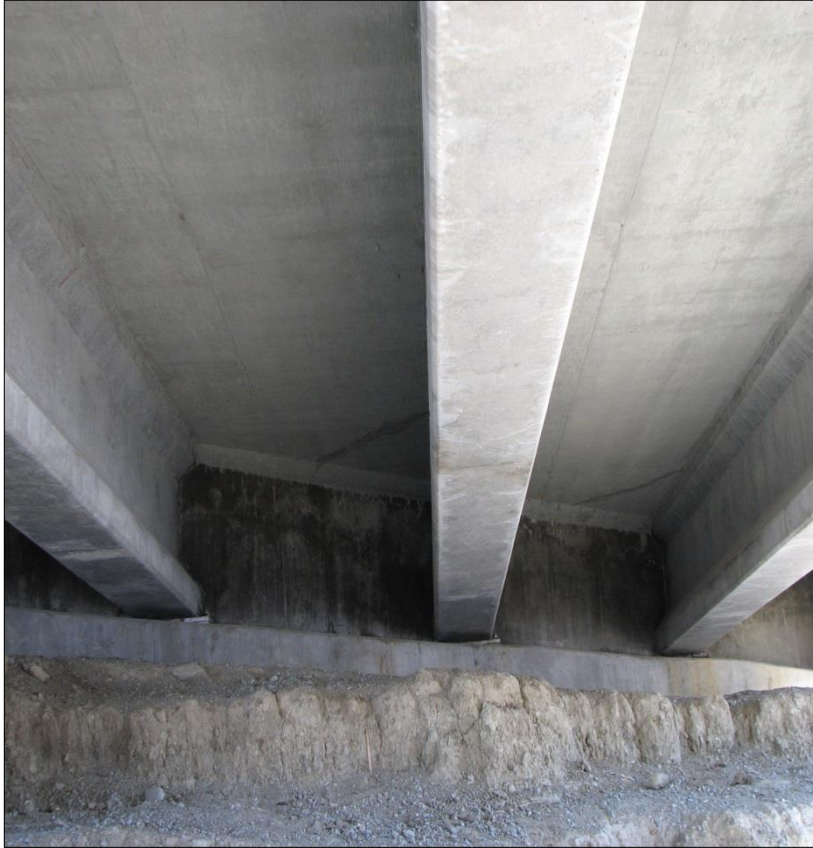
← Example image of full-depth crack, east end of deck; south side.
