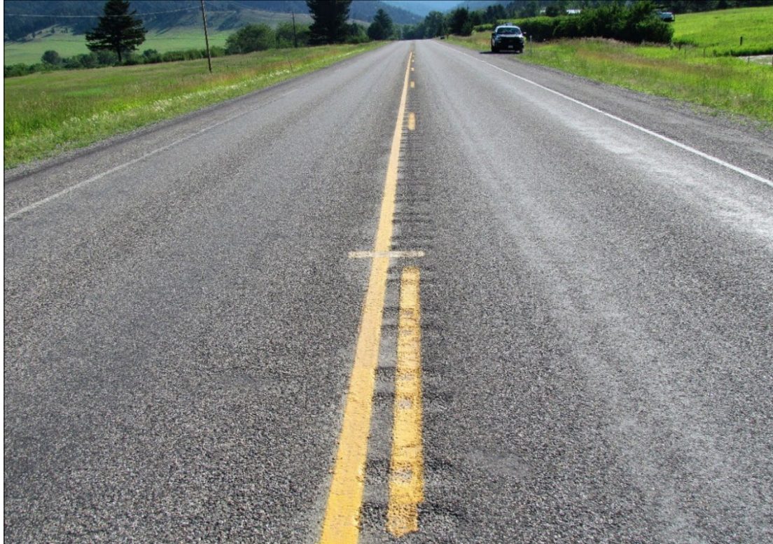
↑ Condition of Jointbond 6 weeks after application.
