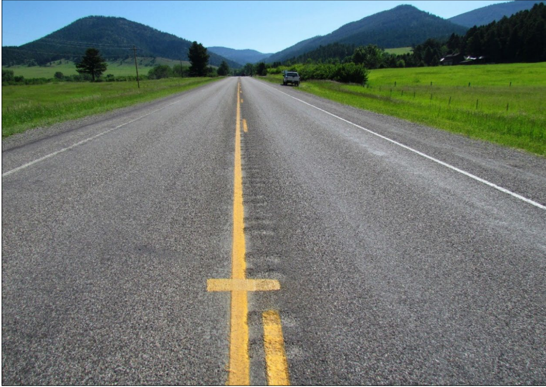
↑ Condition of Jointbond 2 weeks after application.
