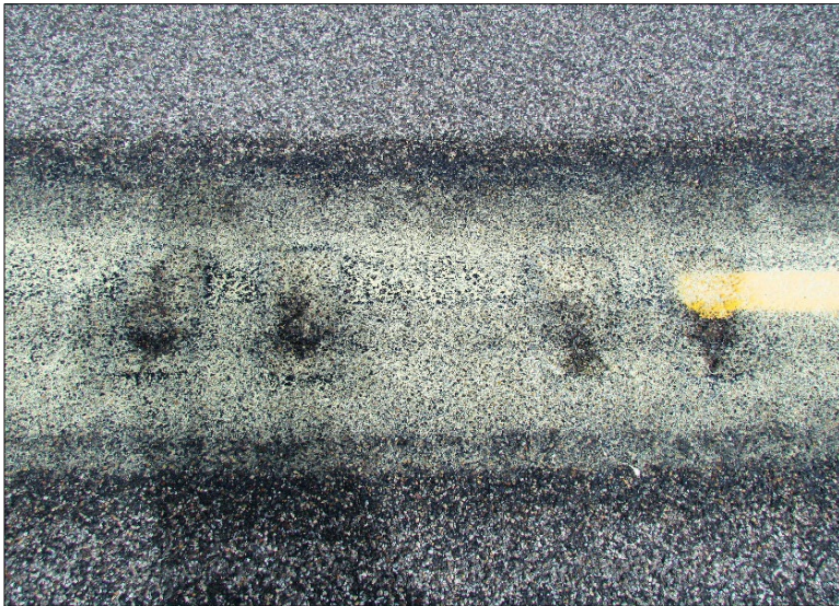
← Close-up of Jointbond showing uniform distribution along the longitudinal paving joint and an approximate width of 1 to 1.5 feet on each side of the joint.
