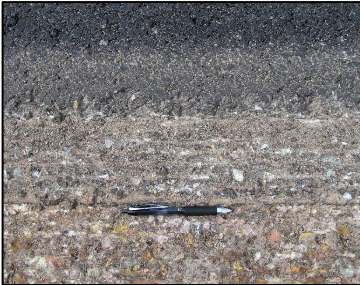
← This image shows the mill pass that has cut into the southbound lane JBAND strip. The pen marks the edge of the JBAND strip.
