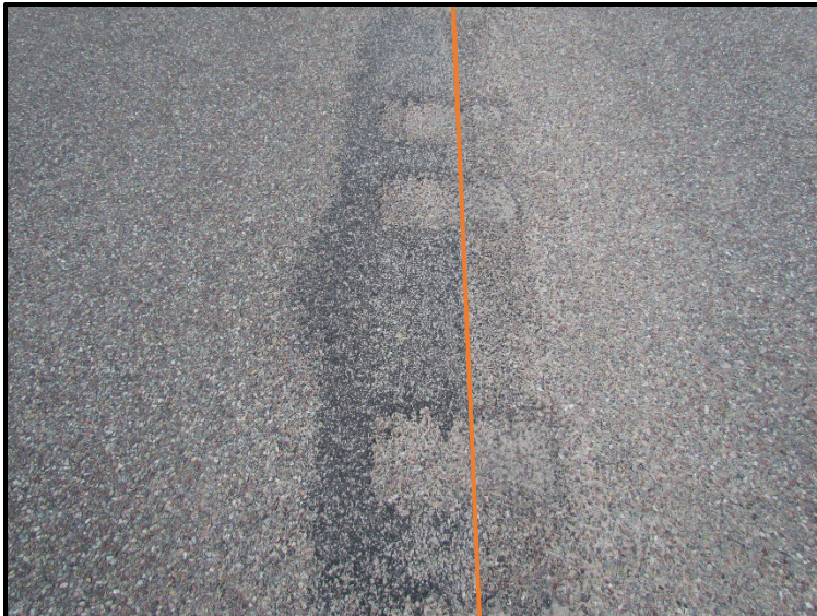
← RP 38.3, close-up. The orange line highlights, most likely, the centerline joint seam.
