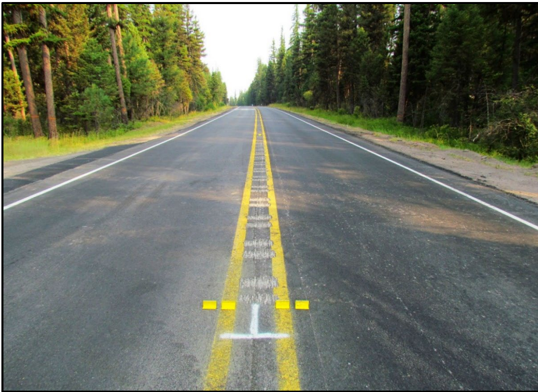
↑ Project with temporary striping and centerline rumble strip. Chip seal was completed in August 2020.
