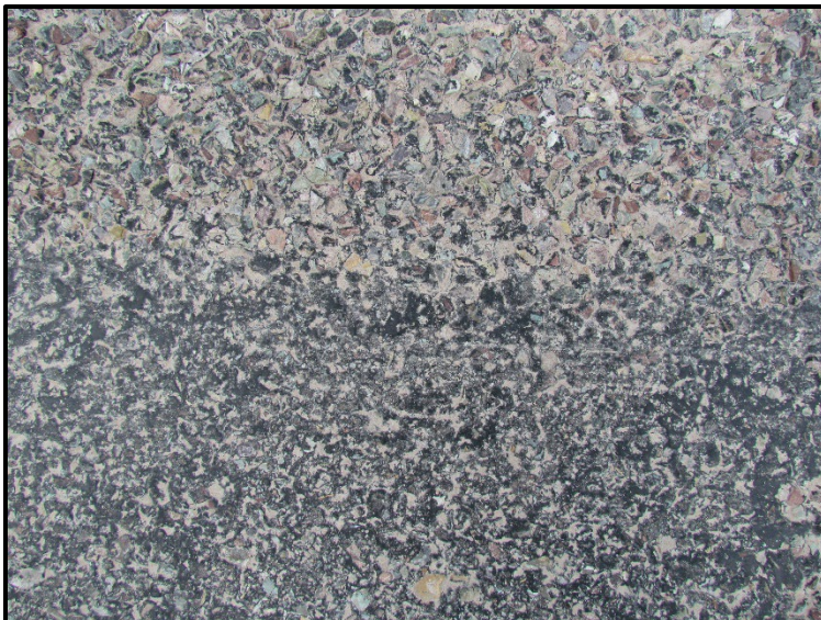
← RP 38.3, close-up. Closer view of the seam from the photo above.
