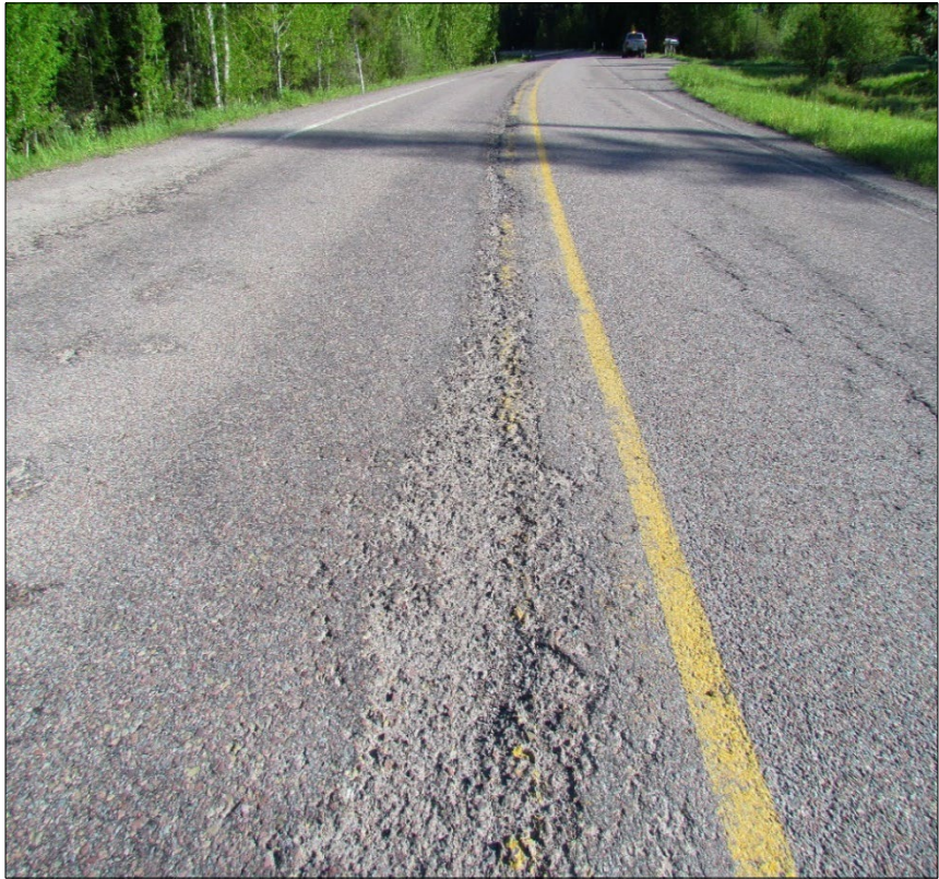
↩️⬇️ Several examples of centerline joint condition prior to start of project. Top image is near RP 32, lower is near RP 43.
