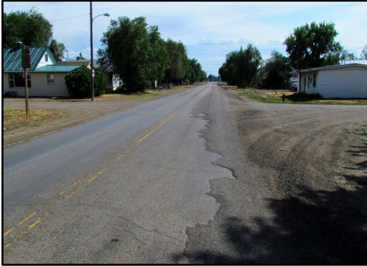
← Representative images of pavement condition prior to reclamation. Areas of visible fatigue, distress, and excessive patching. Area is north end near US Hwy 2 of Sargent St., view south towards town.
