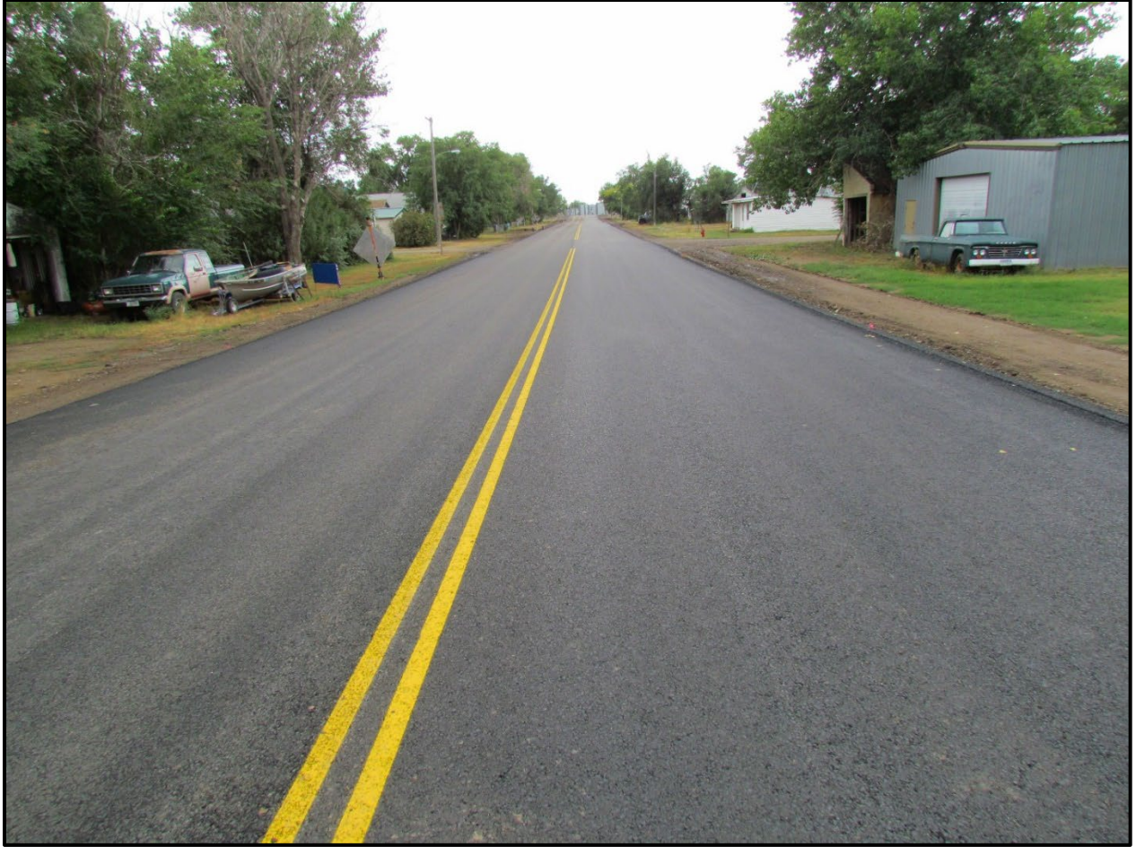
↑ Representative image of completed paving phase of project, Section 6. (Sargent St., view south)
