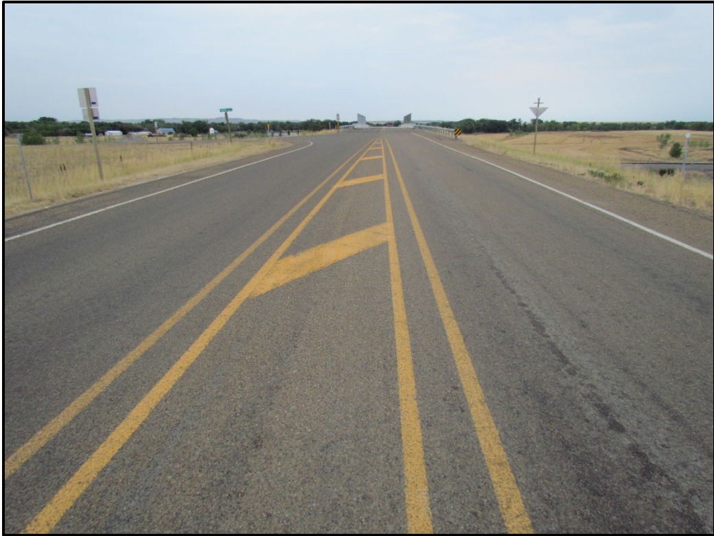
↑ Example of pavement conditions in section 4, view south.
