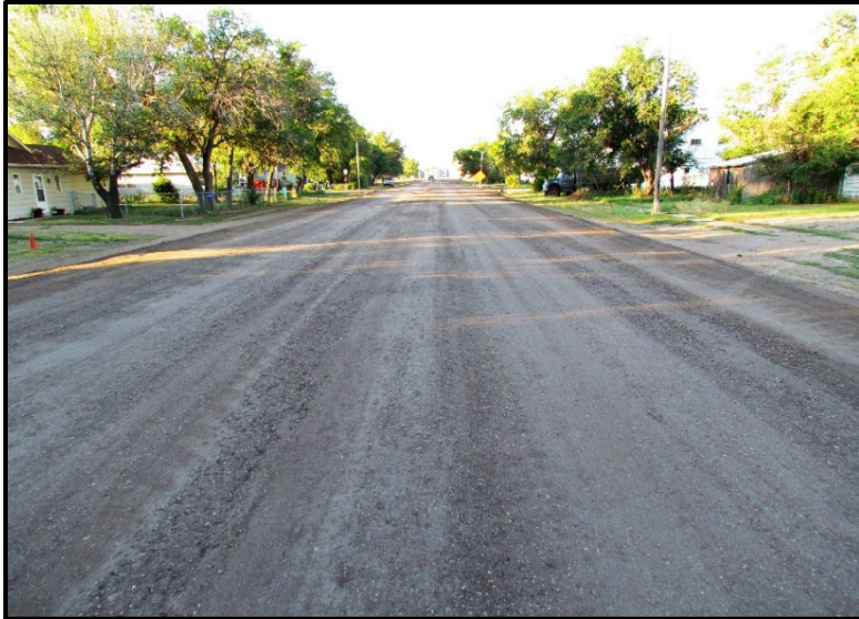
←↓ Representative images were taken several days after stabilization phase was completed. Compaction was completed with a nine-wheel pneumatic roller and drum roller.
