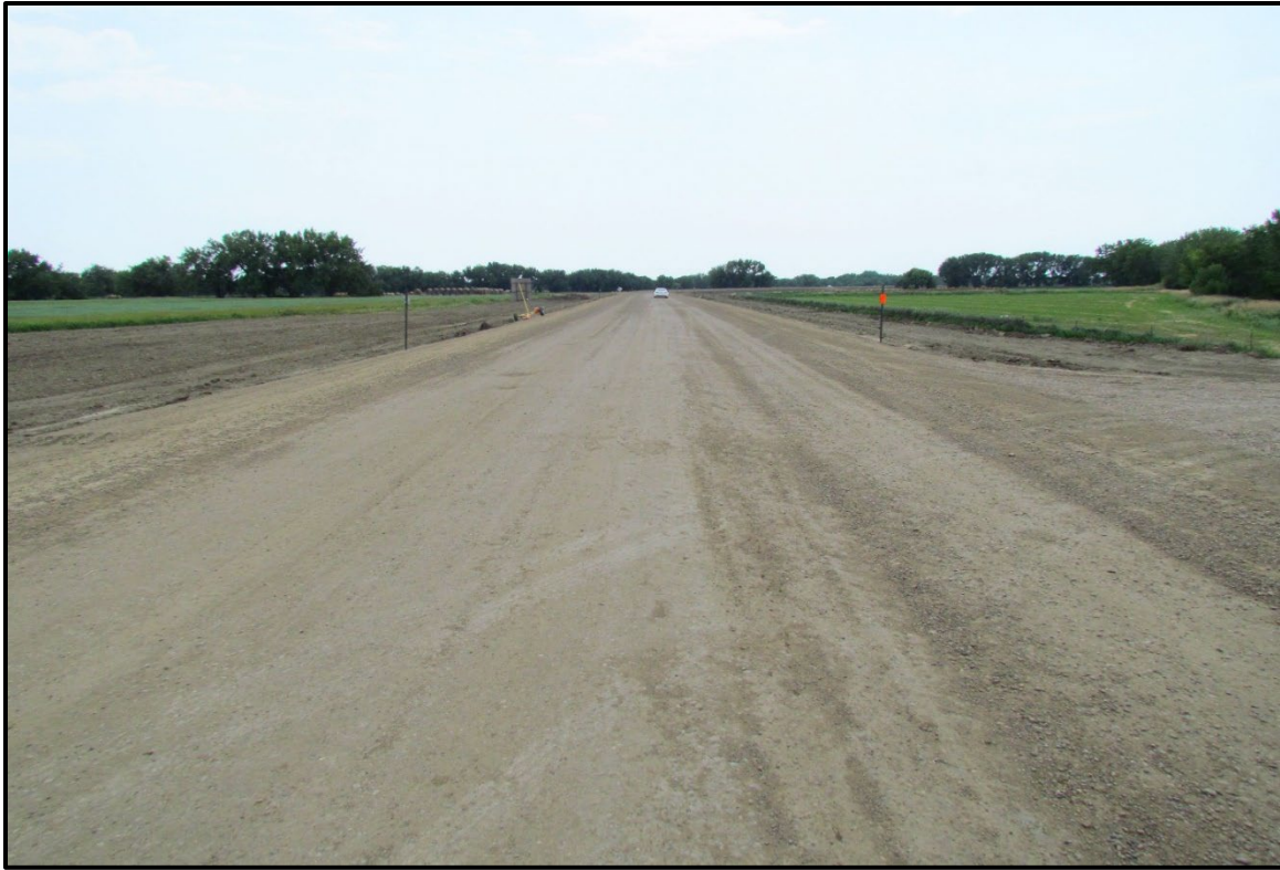
↑ View of treated base approximately two weeks after compaction, Section 1 view south towards Milk River bridge.
