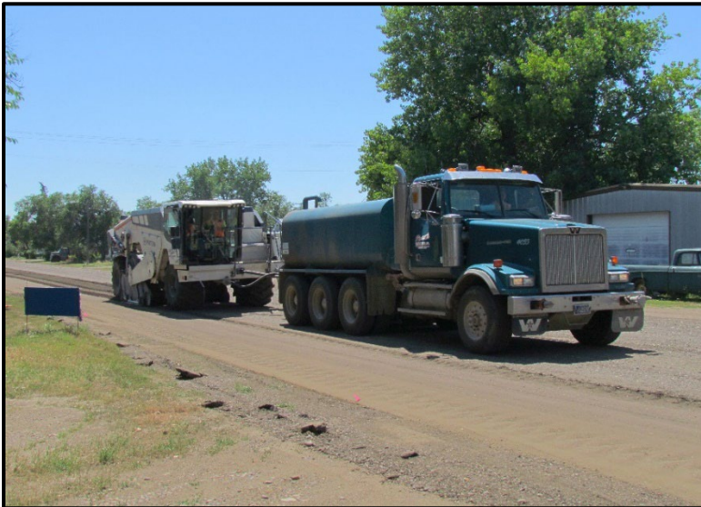
← Additional view of the Base One soil binder mixture in process. The wr250 uses a computer-controlled metering system to ensure a homogeneous mix based on project specifications. The Wirtgen wr250 is connected to the tank truck which doubles as the tow unit. The metering systems automatically adjust mixing ratio as speed varies.
