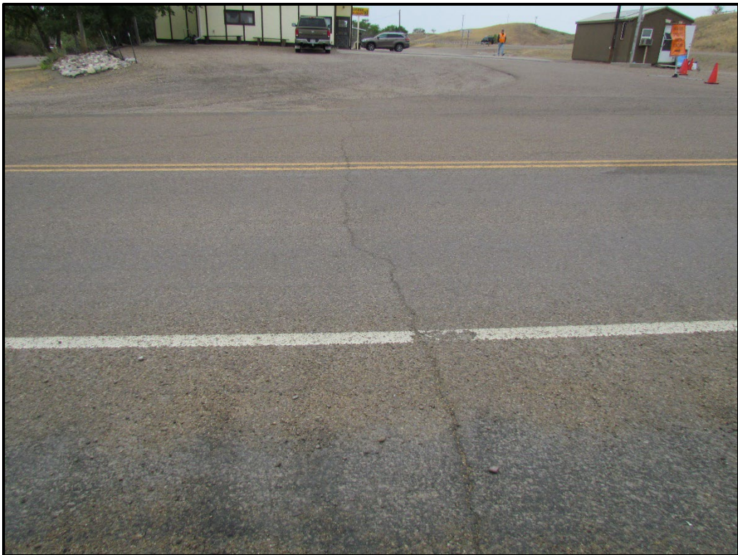
↑ Transverse view of a crack noticed in section 6.
