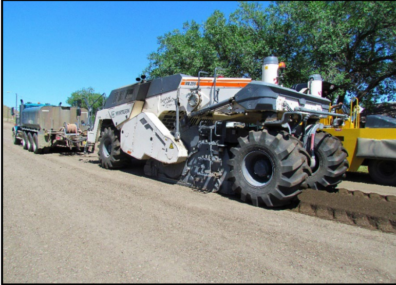
← A high-performance Wirtgen wr250 was utilized on the project for both reclamation of the existing pavement as well as the soil stabilization mixing phase. This image shows the mixing phase (Sargent St.).
