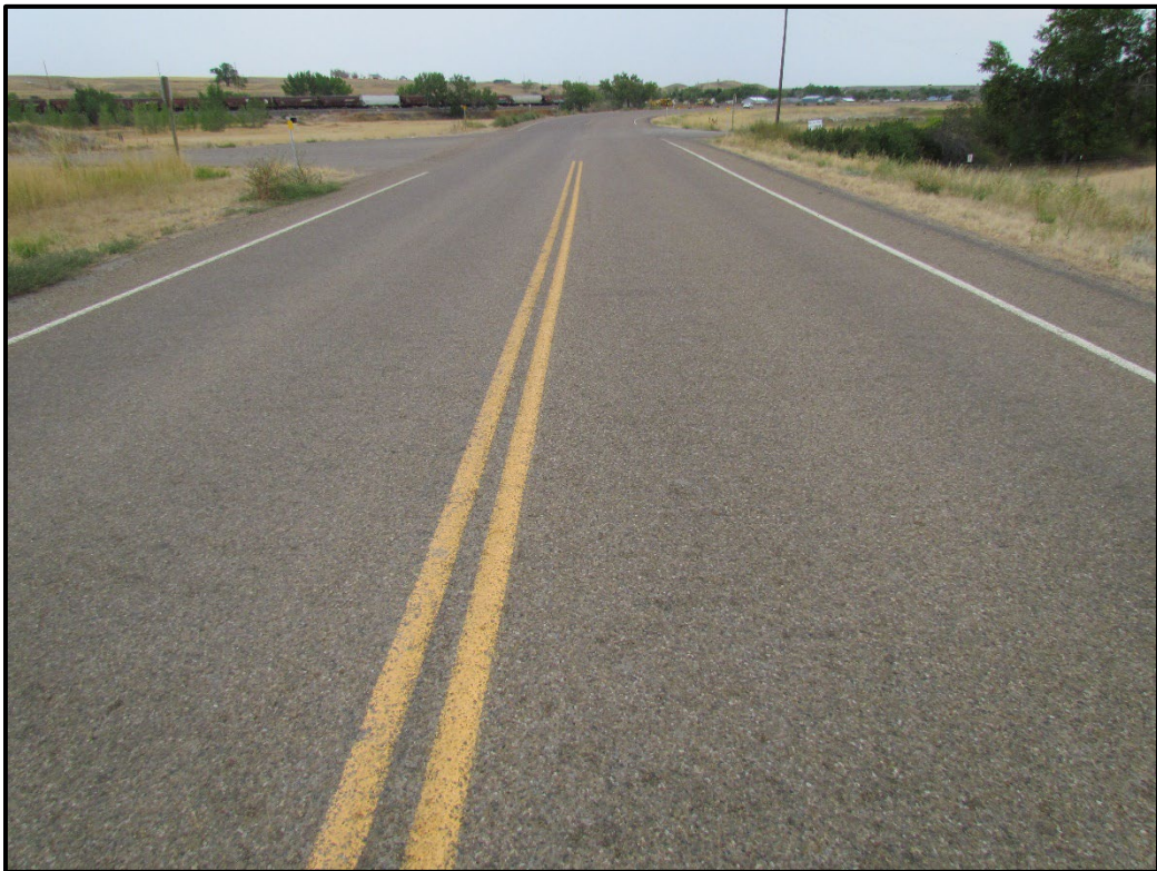
↑ Example of pavement conditions in section 5, view east.
