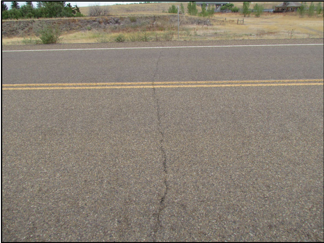
↑ Transverse view of a crack noticed in section 5.
