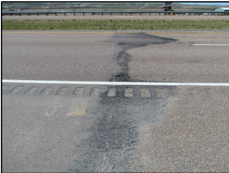
← RP 284, transverse view. As seen, there is some chip loss at the transition joint possibly from snow removal activities.
