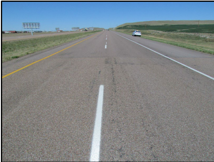
← RP 283, view north. View of the transition from the 3/4" PMS chip seal section to the 3/8" PMS with no chip seal.
