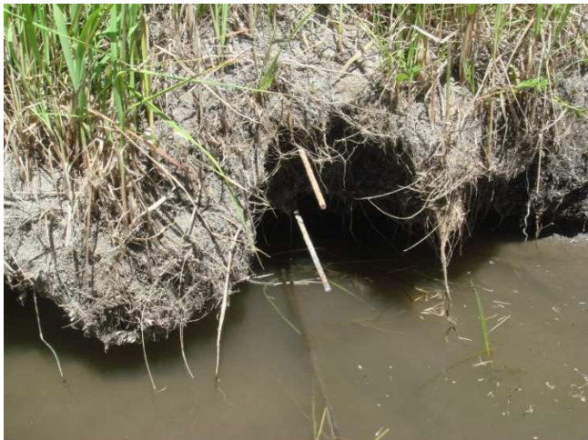
Bank Erosion Pin #1 Taken in 2012
