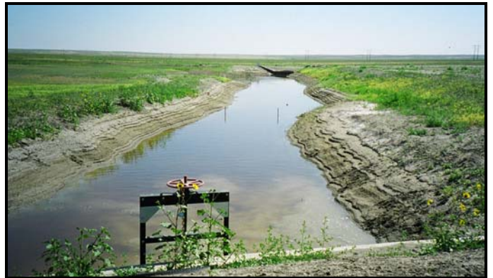
Photo 6: At Photo Point 4 in 40° direction. At inlet control structure looking at diversion structure in background.
