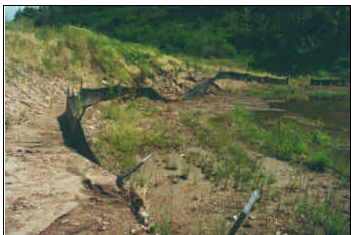
Location: F Photo Frame: 8A Description: Erosion issues below road edge Compass Reading: ~110
