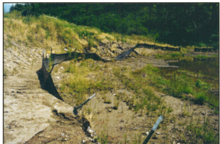
Location: F Photo Frame: 8A Description: Erosion issues below road edge Compass Reading: ~110
