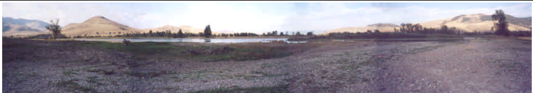
Photo Point No. 10: View looking west; inlet to backwater channel. Area of excavation and grading work, removal of headgate historically controlling the flow of water into remnant backwater channel. Substrate consisting of cobbles and gravels, low vegetation cover, mapped as Waters of the US jurisdiction.
