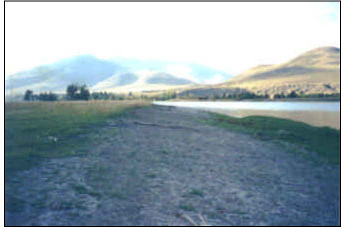
Photo Point No. 12: View looking northwest along Flathead River. Area of excavation and grading work to remove historic berm along north boundary of site.
