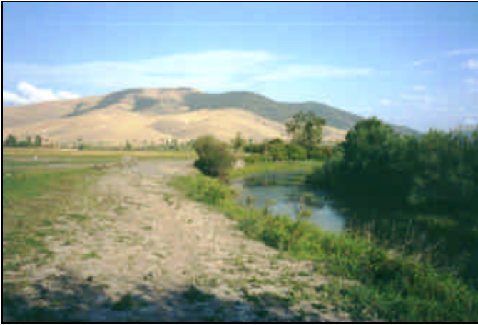
Photo Point No. 7: View looking east; areas of excavation and grading along backwater channel, removal of berm along north edge.
