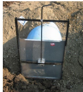
Slide Gate in Field
