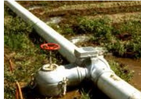
Irrigation Hydrant Connected to Gated Irrigation Pipe
