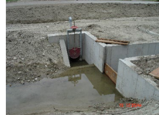
Check Structure with Gate
