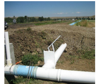
Gated Pipe with Slide Gate
