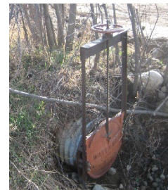
Cast Iron Wheel Gate
