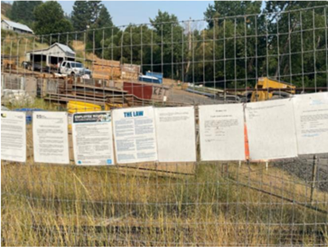
Required notices and posters are laminated and affixed to a fence with zip ties.
