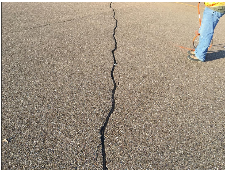
AP05-06: L&T Cracking
