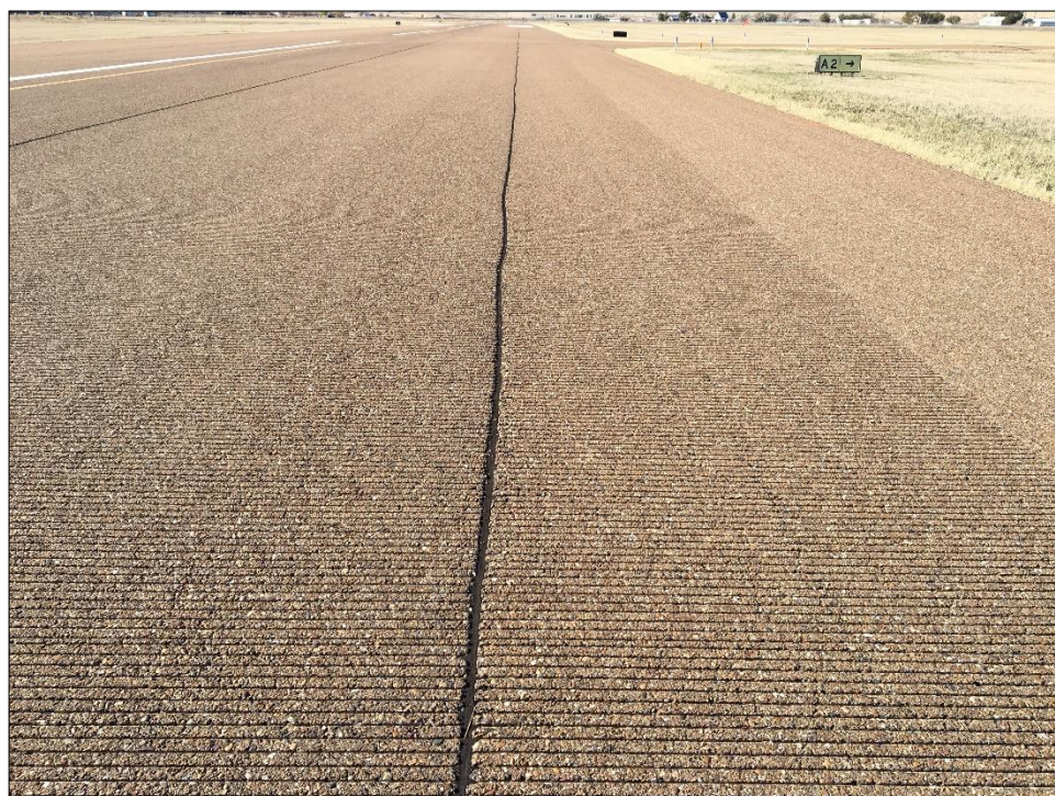
RW11-11-65: L&T Cracking
