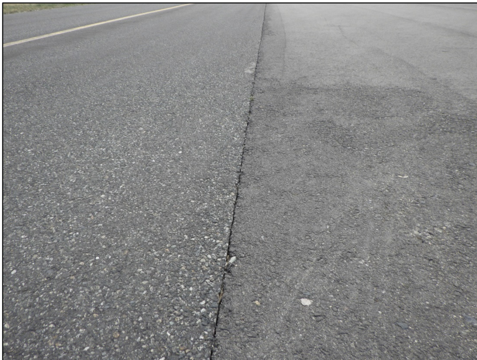
TW12-03: L&T Cracking
