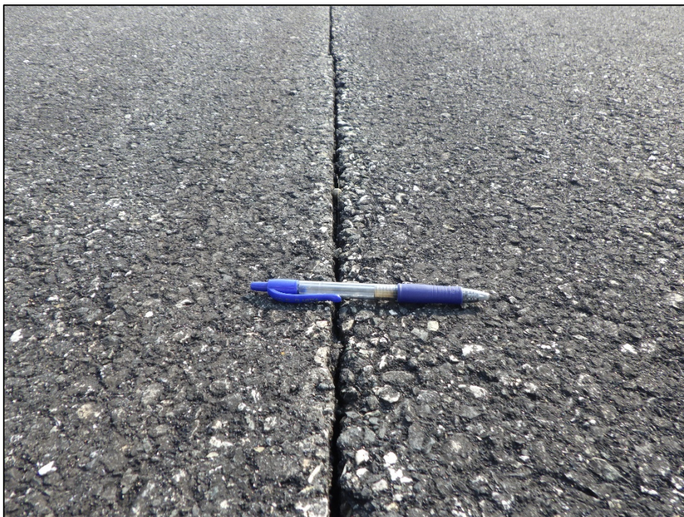
RW17-11-56: L&T Cracking
