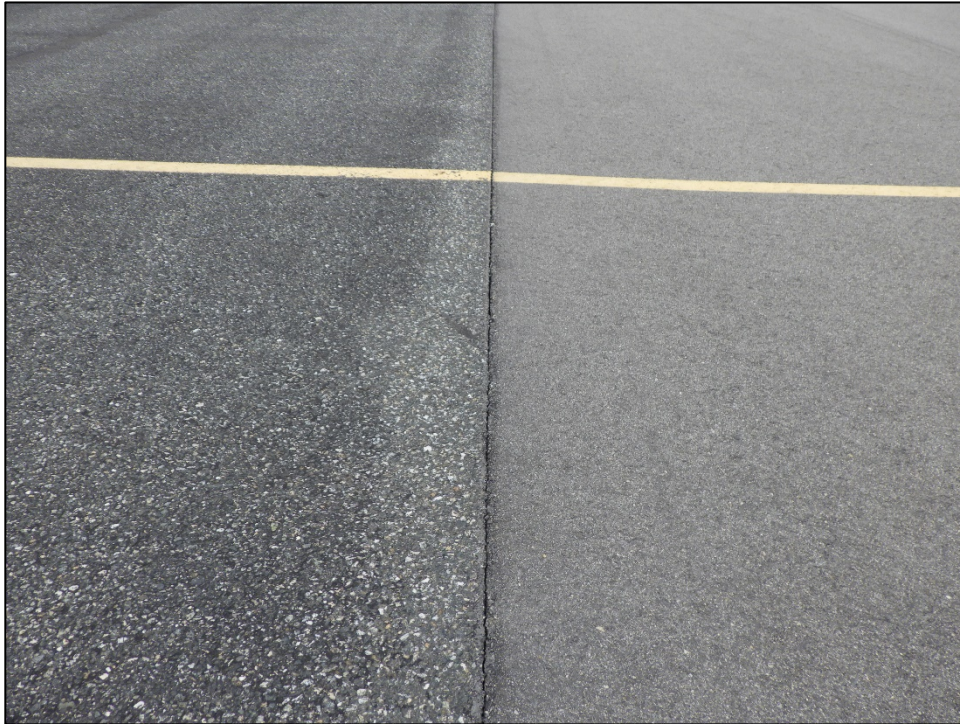
AP02-04: L&T Cracking
