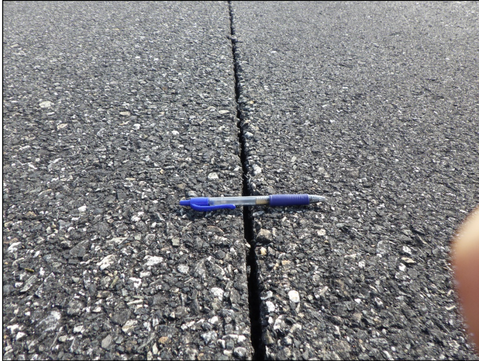
RW17-11-23: L&T Cracking
