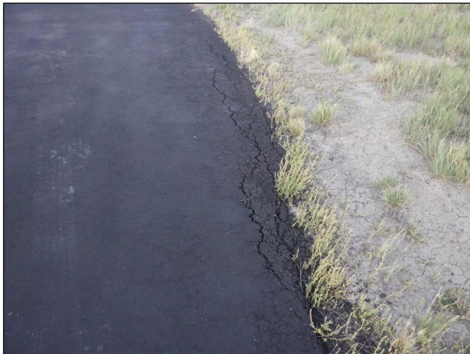
TW17-06: L&T Cracking
