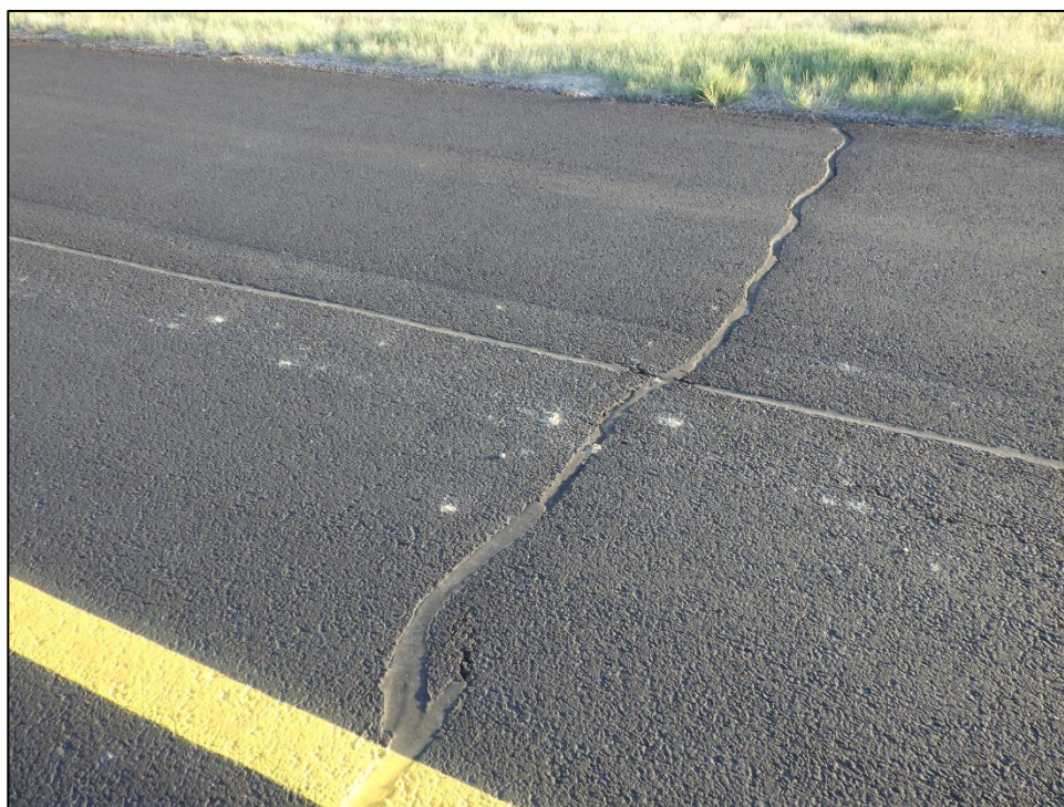
TW21-11: L&T Cracking
