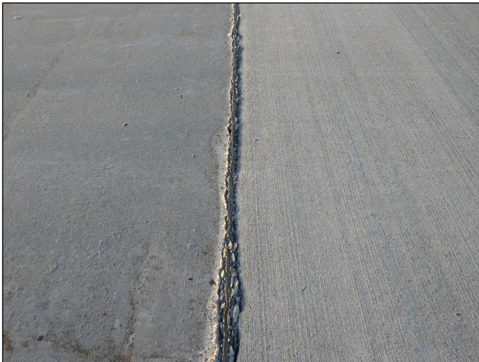
AP22-02: Joint Spalling
