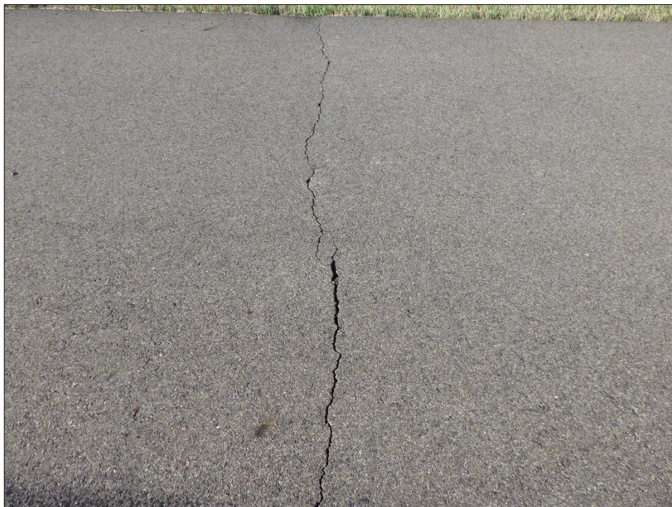
RW12-11-31: L&T Cracking
