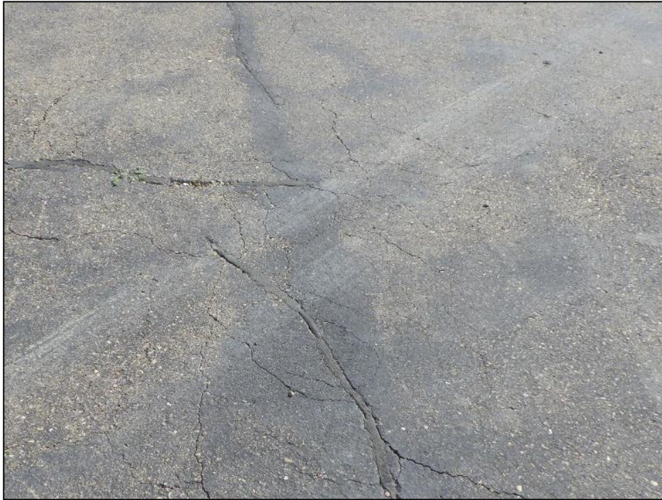
TW11-04: Alligator Cracking
