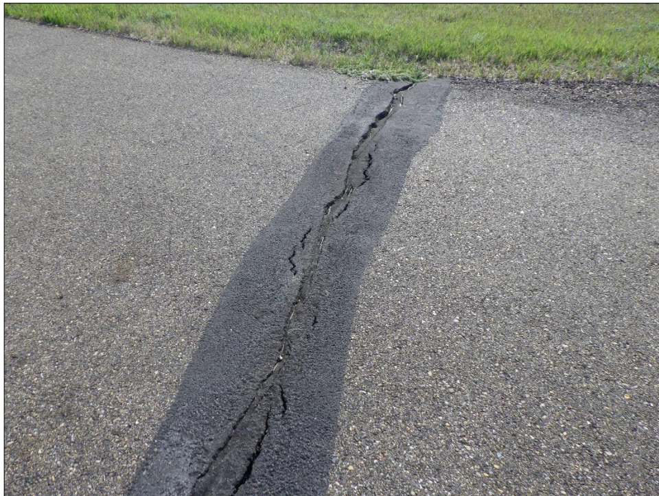
TW13-02: L&T Cracking
