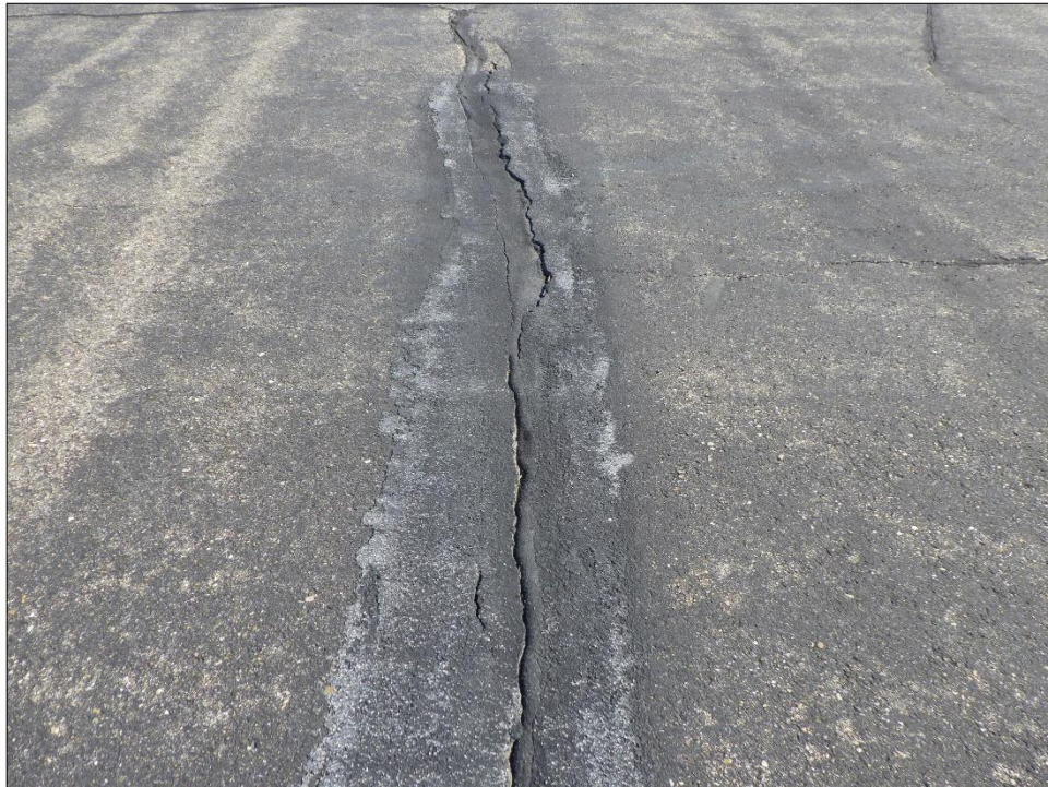
AP11-01: L&T Cracking
