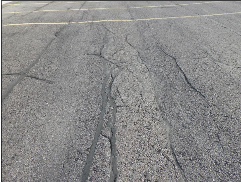
AP11-34: Alligator Cracking
