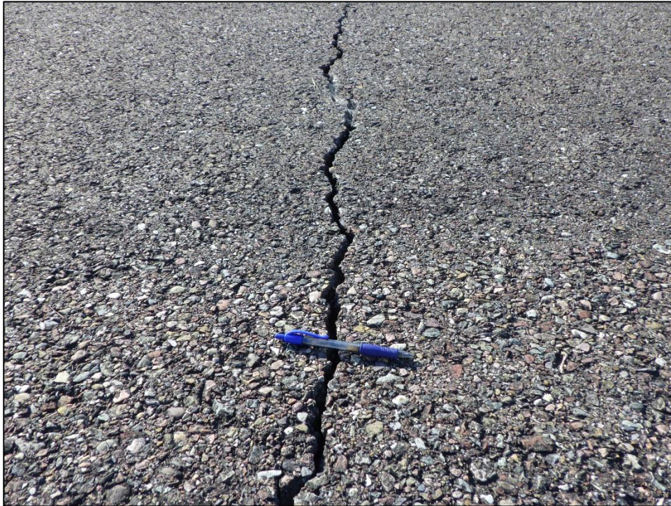
TW11-26: L&T Cracking
