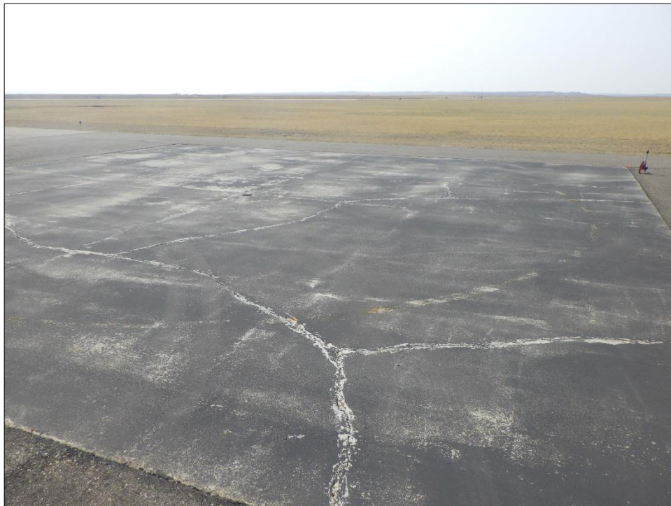
AP05-01: Shattered Slab/Intersecting Cracks
