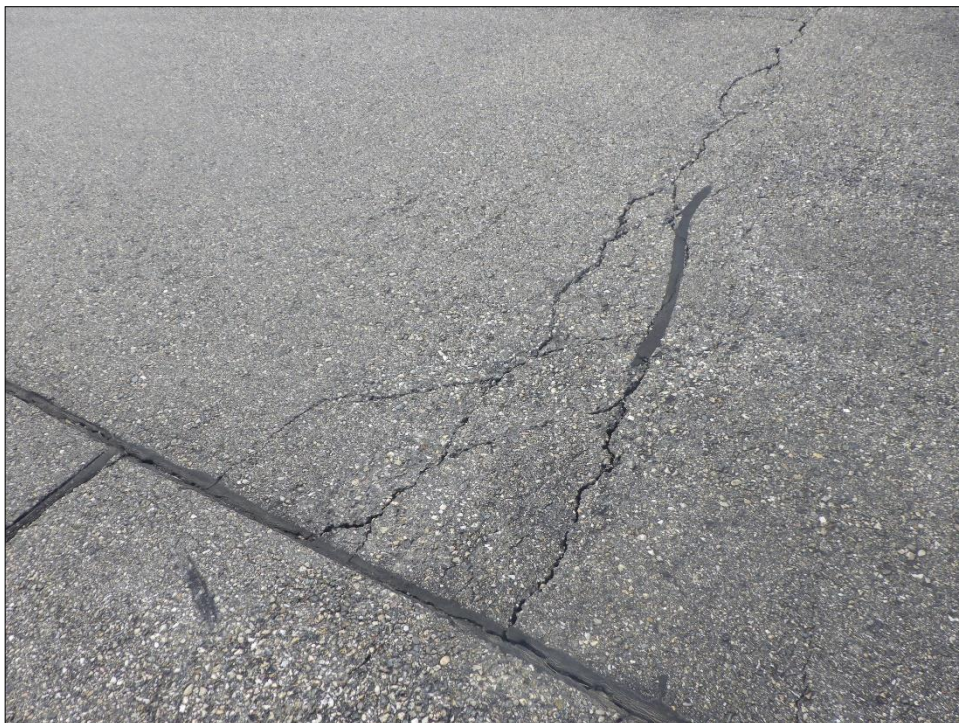
AP04-04: Alligator Cracking
