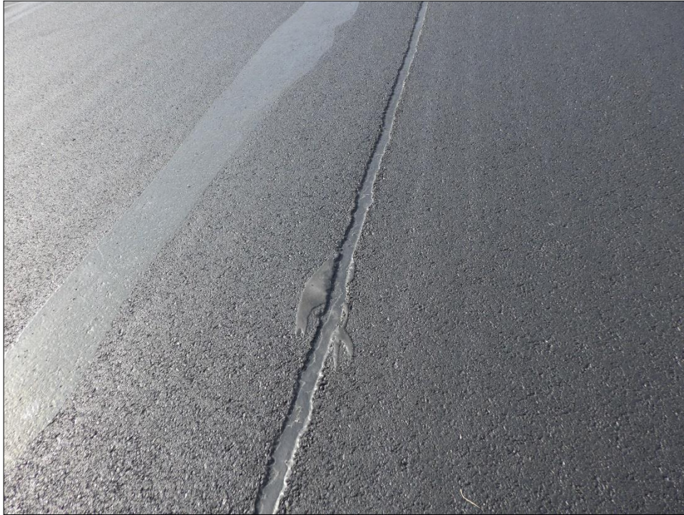
AP01-09: L&T Cracking
