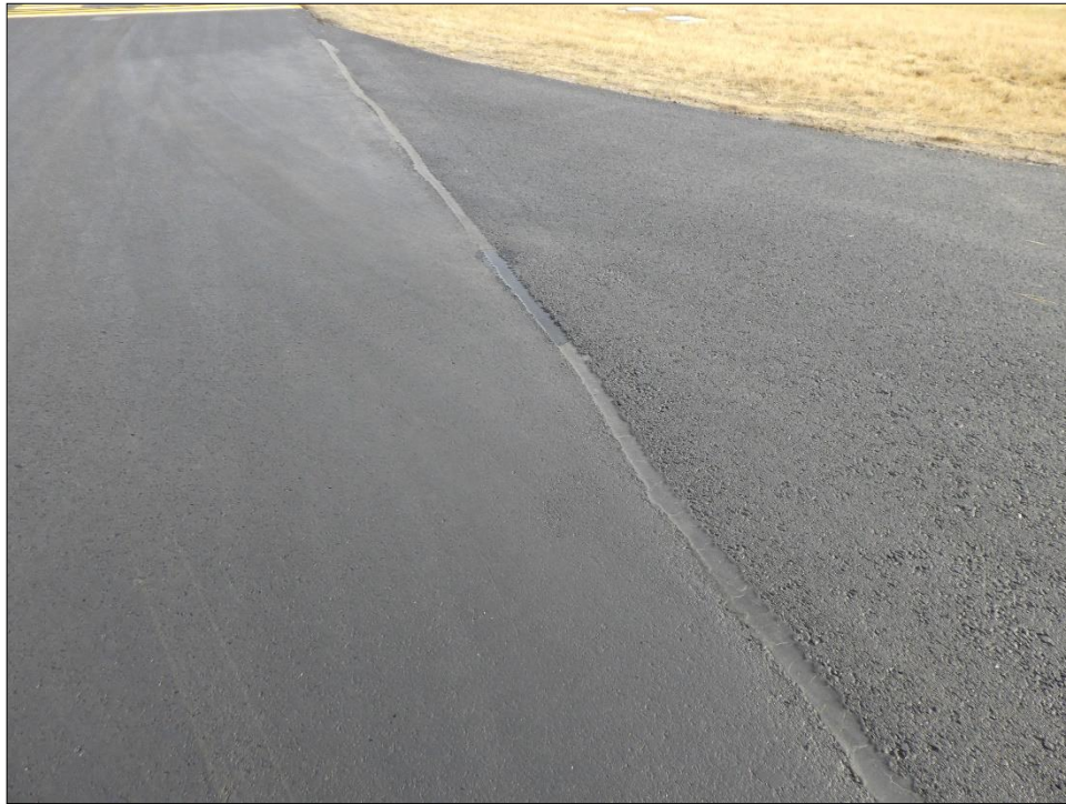
TW01-12: L&T Cracking
