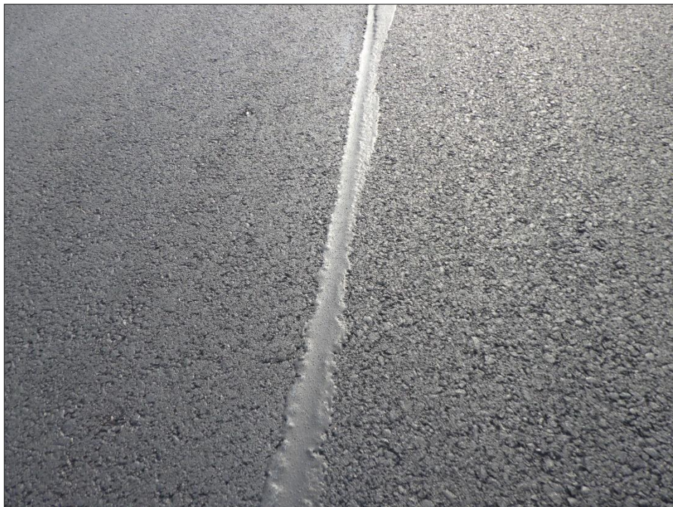
RW08-01-56: L&T Cracking
