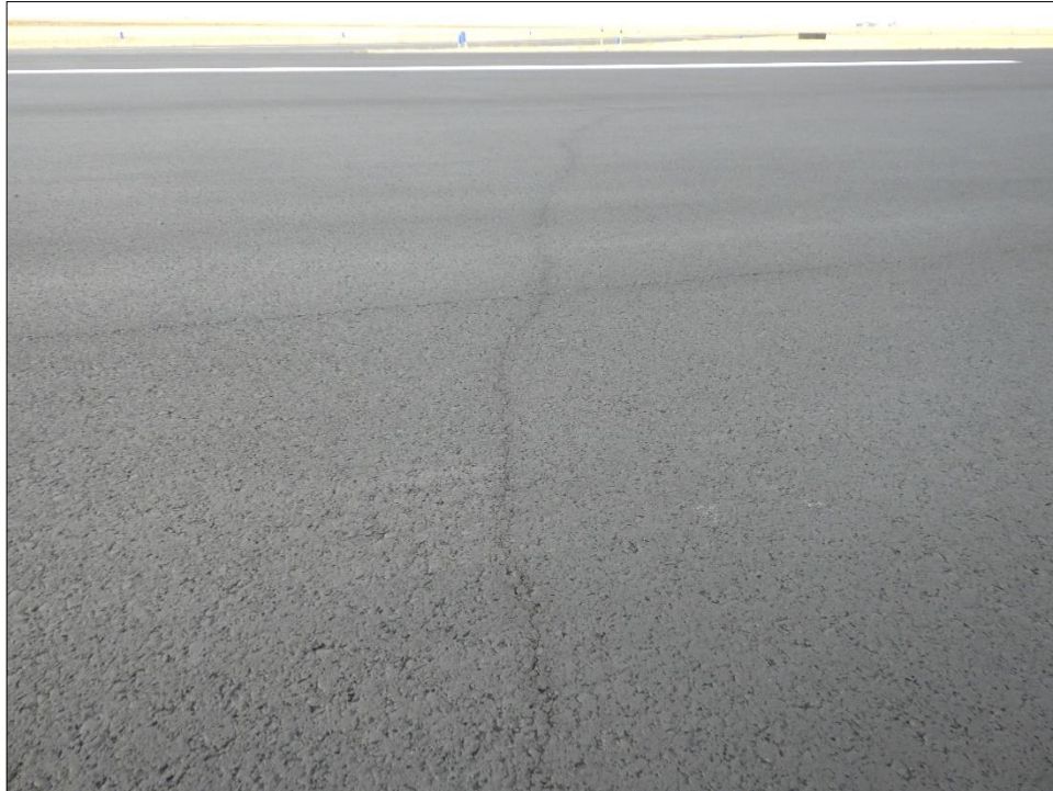
RW08-01-06: L&T Cracking
