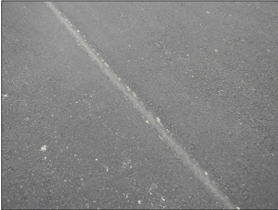
RW05-11-10: L&T Cracking
