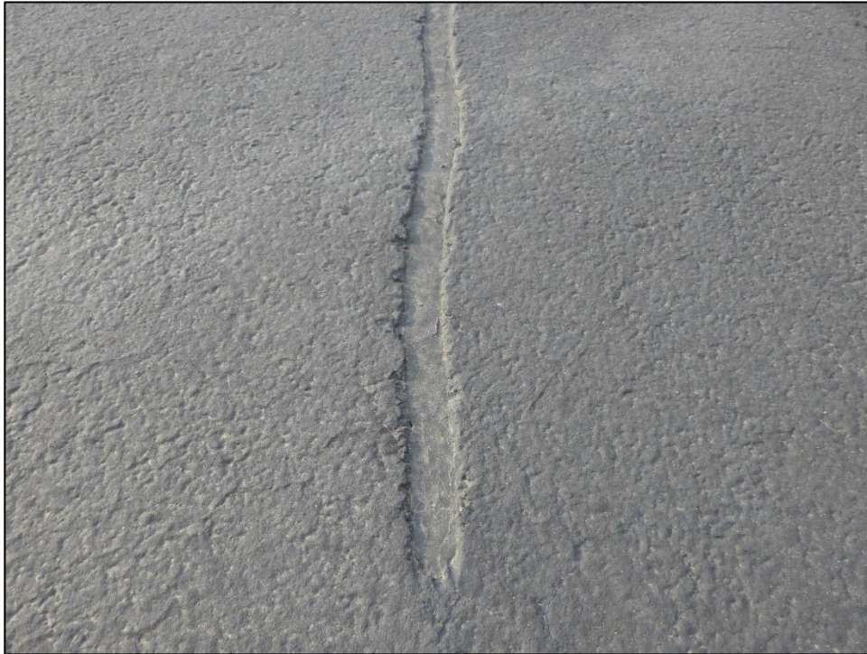
AP11-14: L&T Cracking
