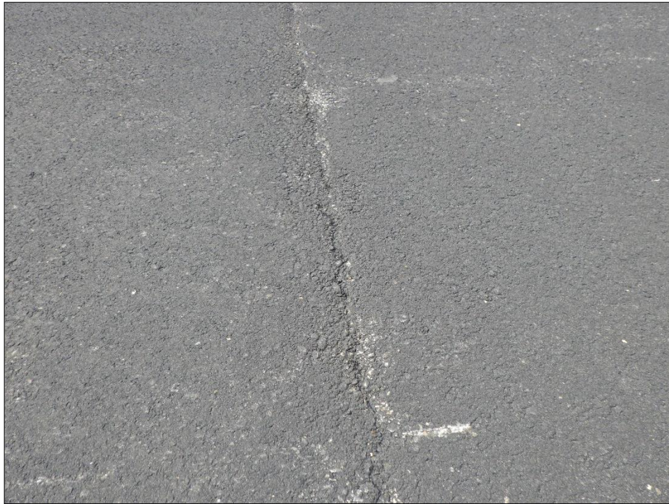
AP03-10: L&T Cracking
