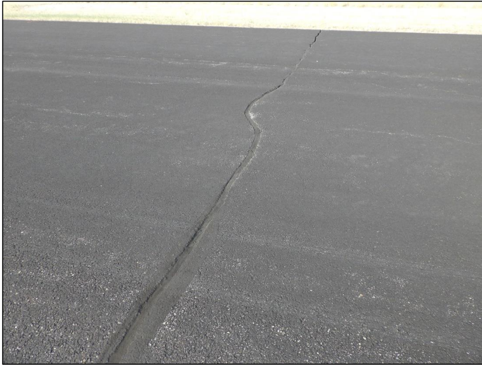
RW17-03-86: L&T Cracking
