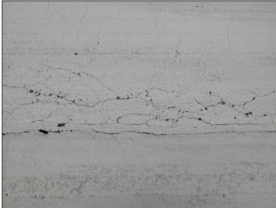
RW17-03-02: Alligator Cracking
