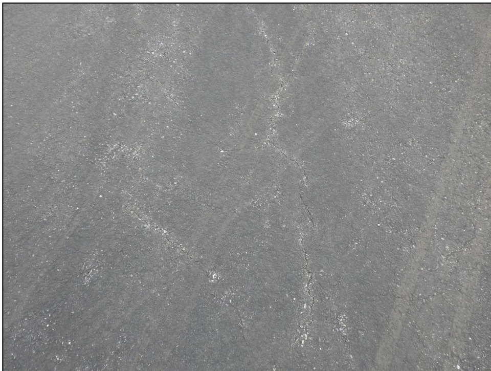
AP04-09: L&T Cracking
