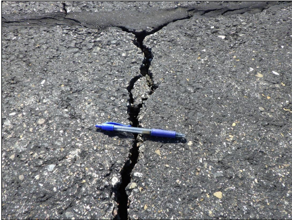
RW06-03-35: L&T Cracking
