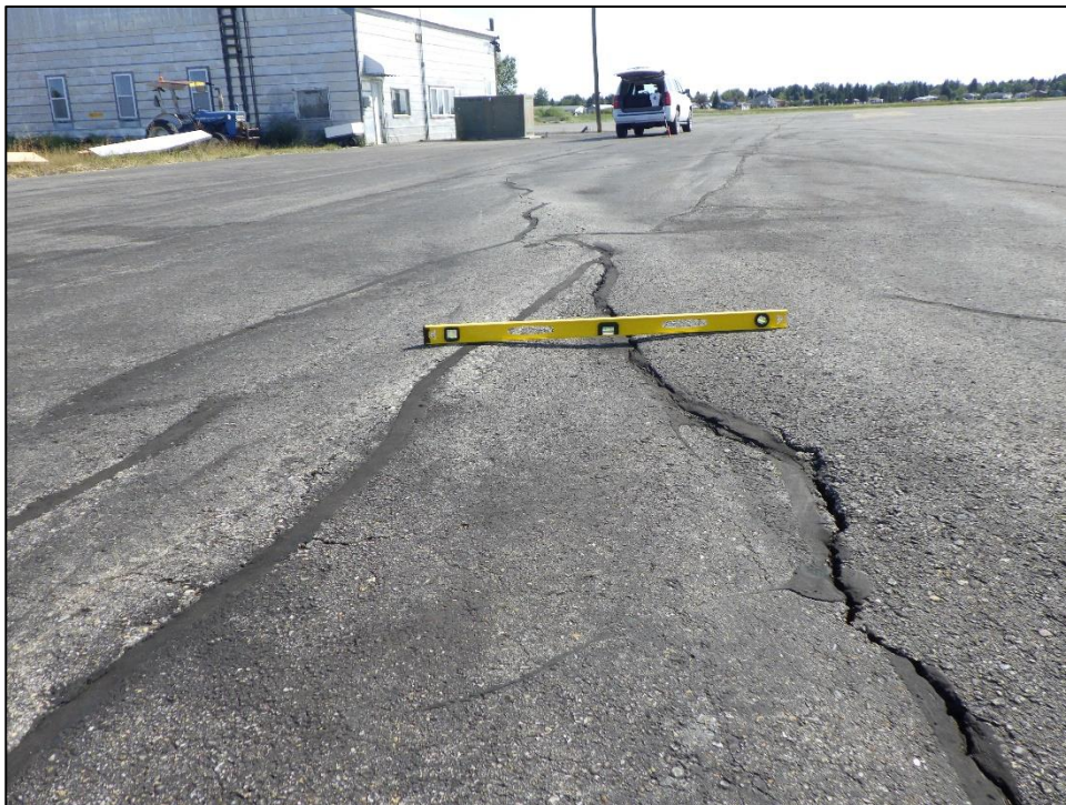
AP01-21: L&T Cracking
