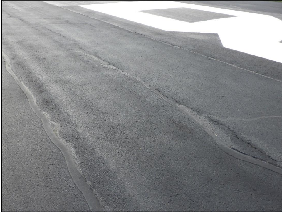
RW08-01-01: L&T Cracking
