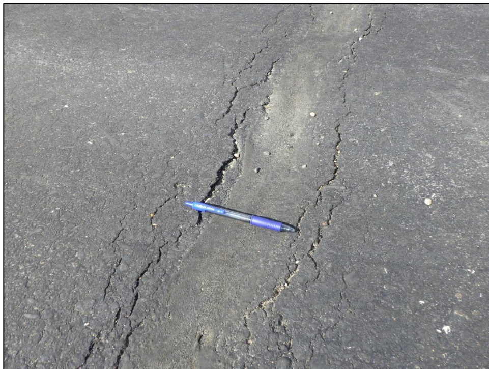
AP05-07: L&T Cracking
