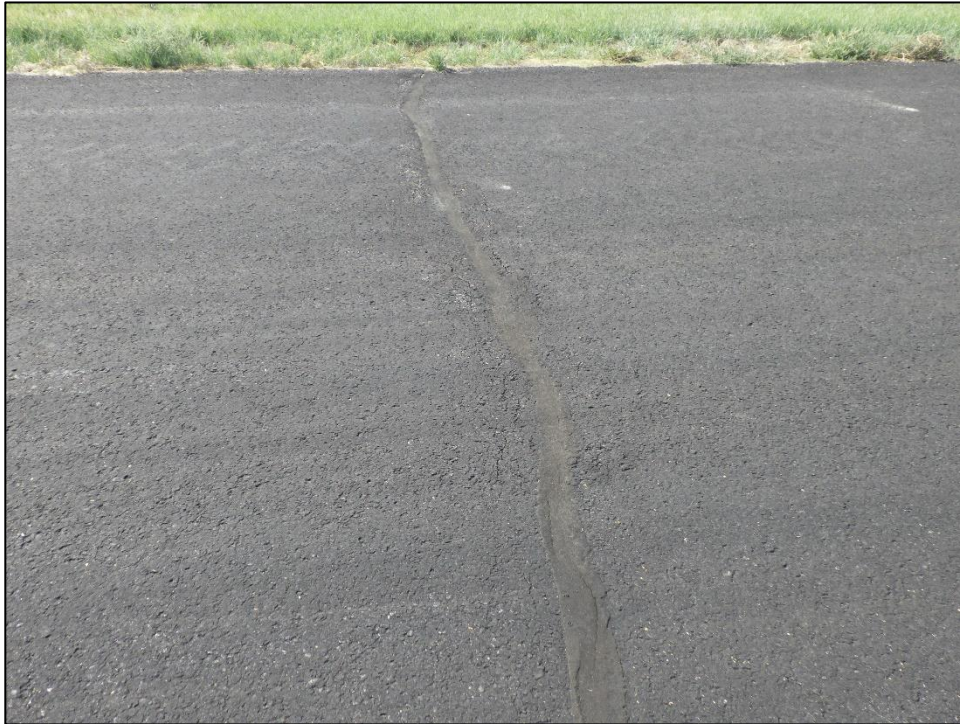
TW02-01: L&T Cracking
