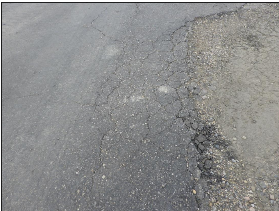
TW03-02: Alligator Cracking
