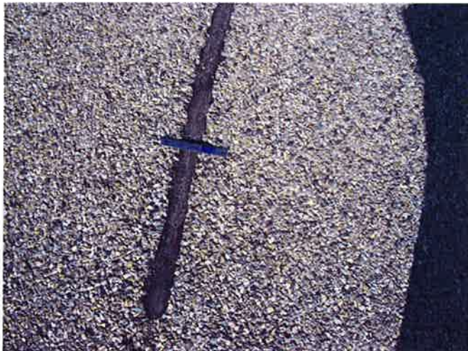
T-2, Surface detail cracking
