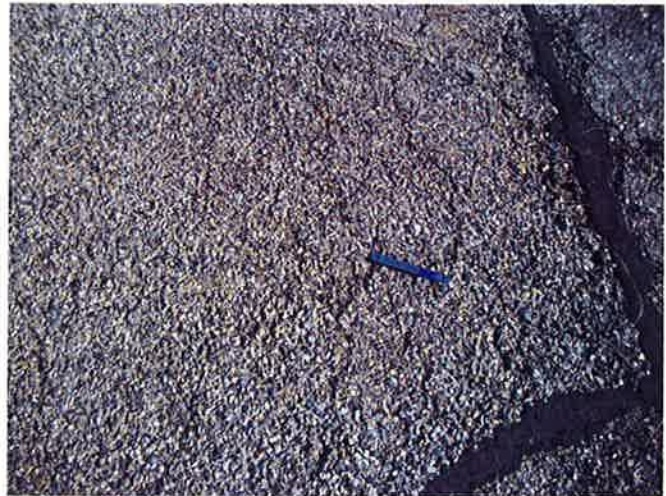
A-1, Surface detail alligator cracking
