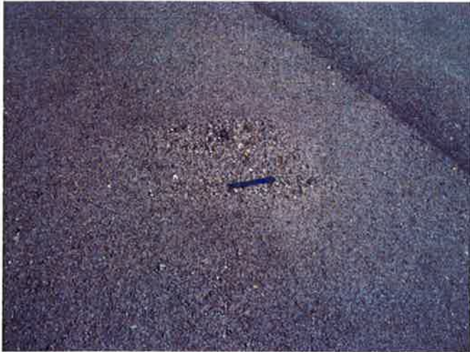
R-12, Surface detail raveling from snow plow
