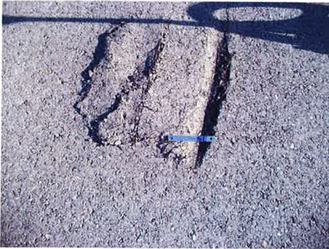
A-11 , Surface damage from helicopter skids
