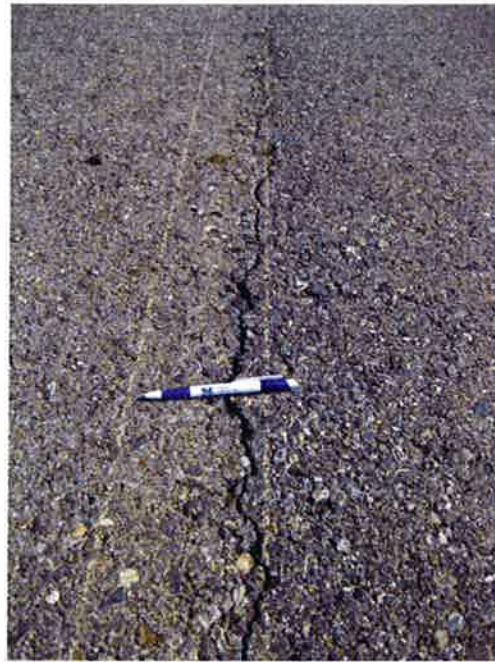
T-1, Surface detail with crack
