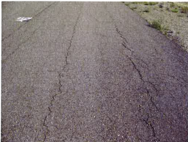
R-1, Surface detail with cracks
