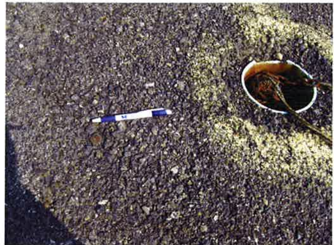
A-1, Surface detail with raveling
