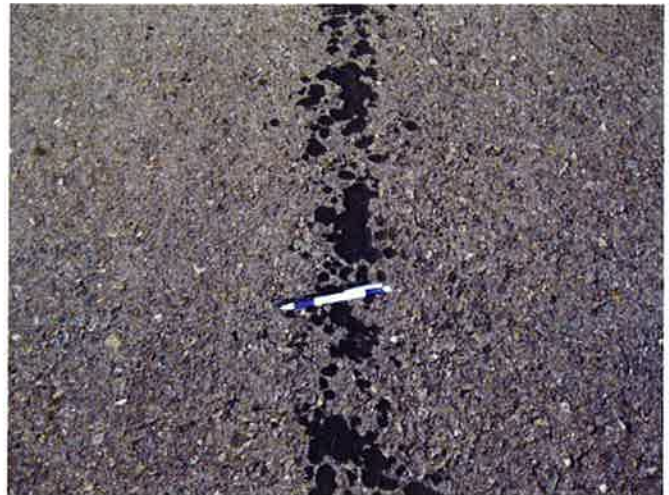
R-1, Surface detail with bleeding
