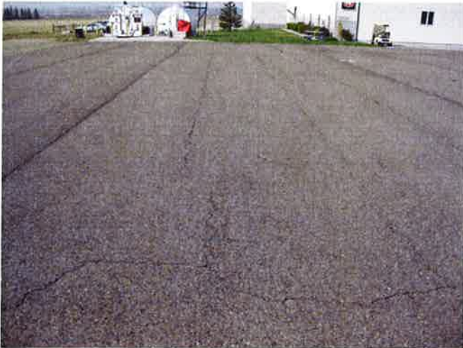
A-1, Surface detail with cracks
