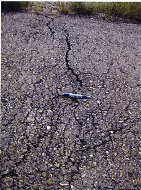
T-1, Surface detail with depression and cracks
