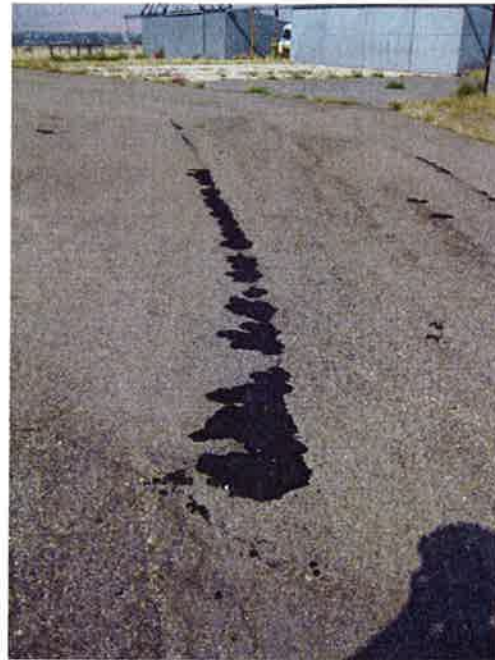
A-1, Surface detail with bleeding
