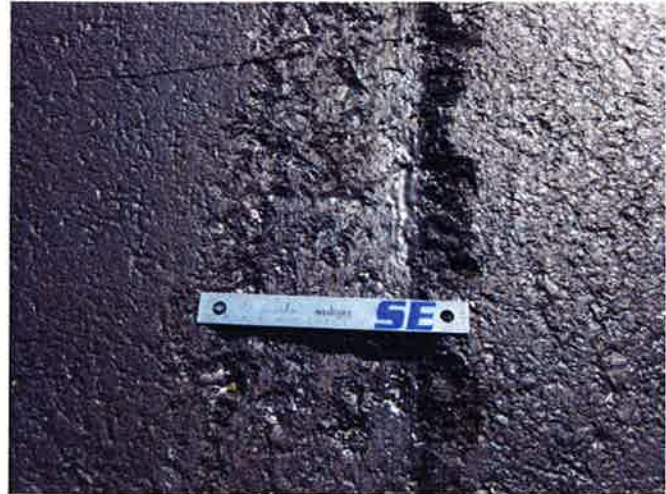
T-3 , Surface detail with depression
