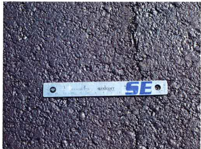
R-1, surface detail with crack
