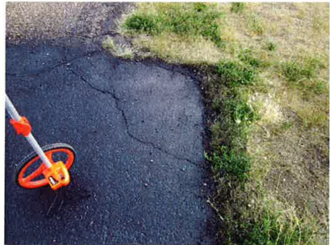
A-1, Surface detail with cracks
