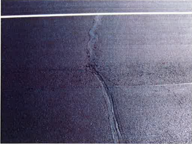
R-1 , Surface detail with cracks
