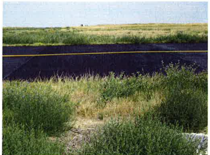
T-2 , surface detail with patching
