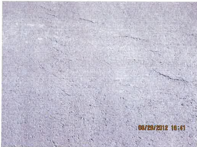
R-1, Surface detail with cracking
