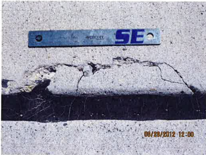
A-2, Surface detail with spalling
