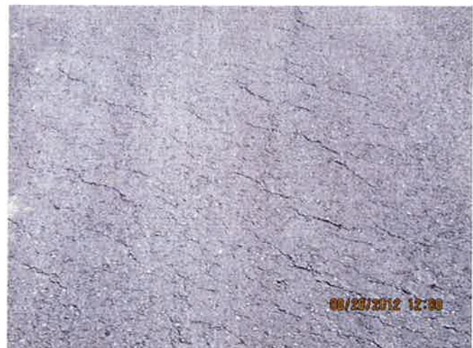
T-1, Surface detail with cracking
