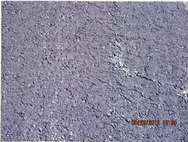
R-2, Surface detail with cracking
