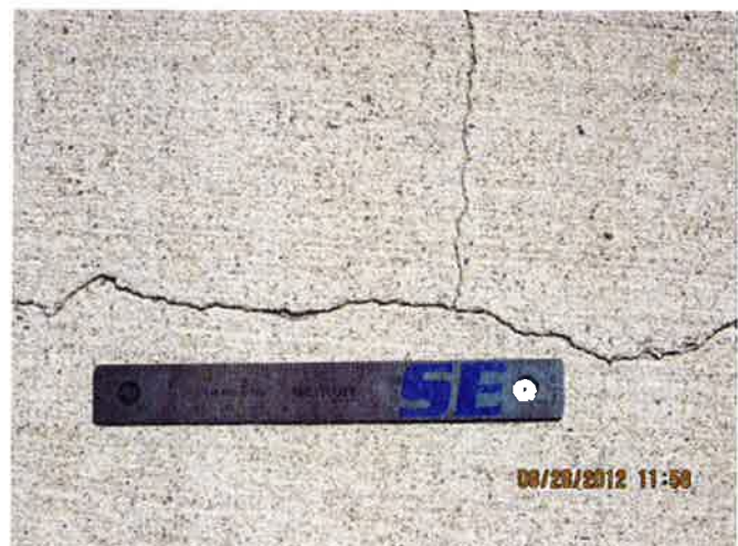
A-2, Surface detail with crack
