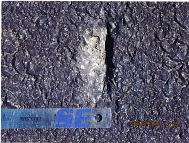
T-2, Surface detail with depression
