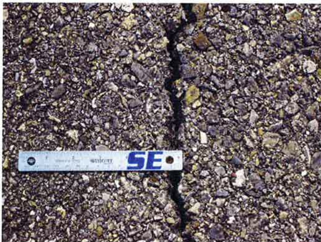
R-3, Surface detail with crack
