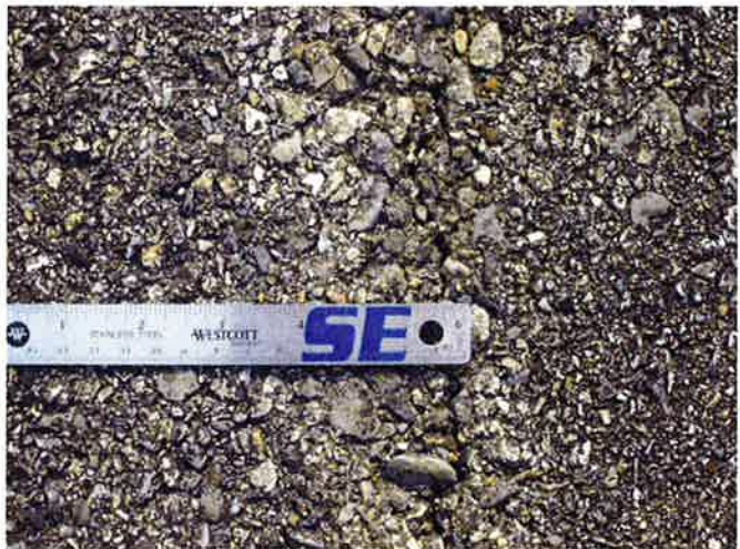
R-2, Surface detail with crack
