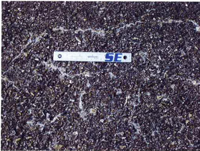
R-2, Surface detail with cracking
