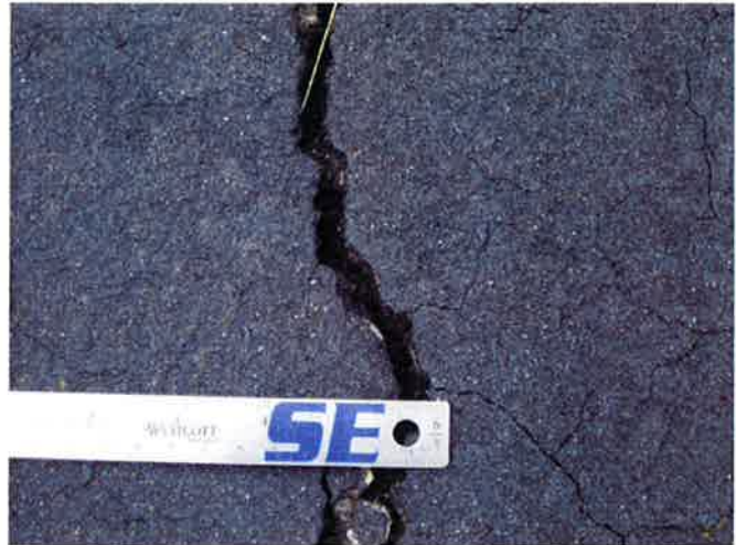
A-2, Surface detail with crack
