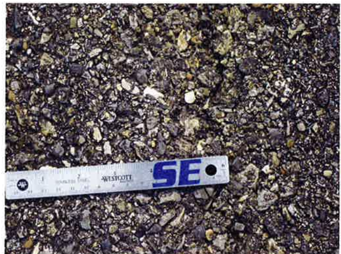
R-3, Surface detail with crack
