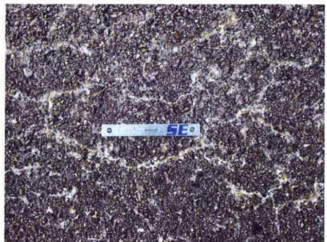
R-3, Surface detail with cracking
