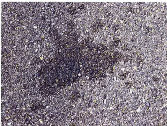
T-2, Surface detail with oil spill
