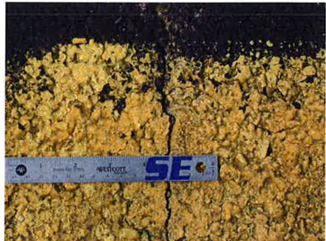
T-2, Surface detail with crack
