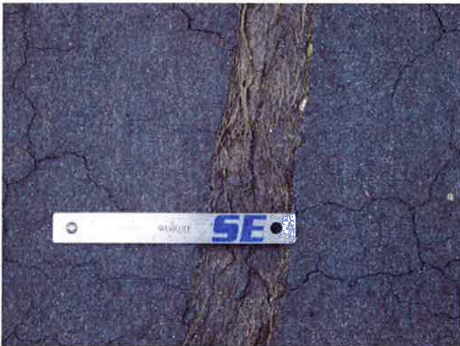
A-2, Surface detail with cracking
