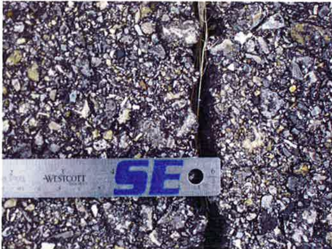
T-2, Surface detail with crack 2
