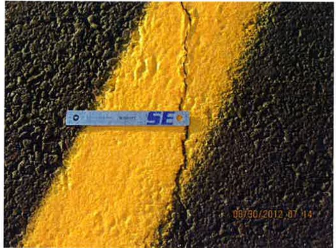
T-5, Surface detail with crack
