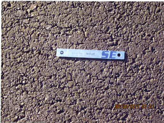
T-5, Surface detail with cracking
