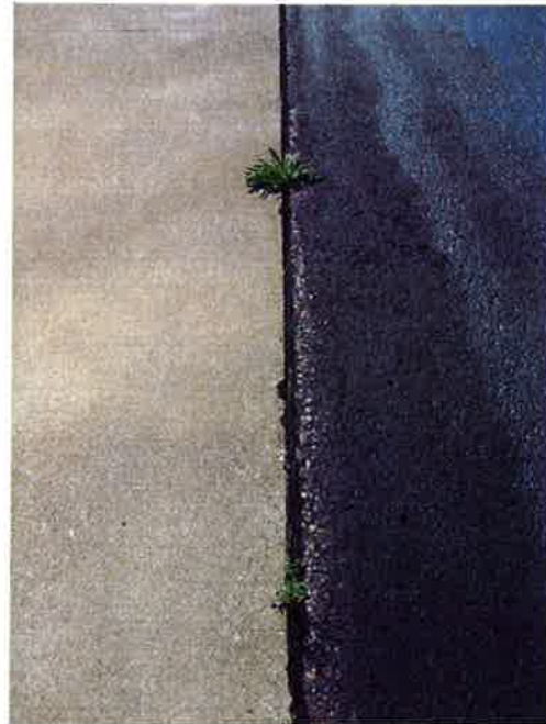
A-2, Surface detail with crack
