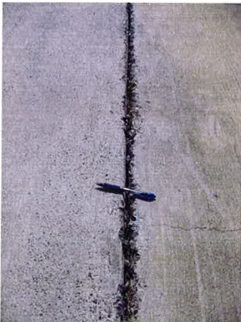
A-5, Surface detail with spalling
