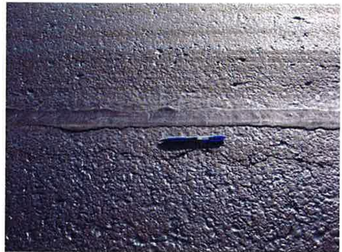
R-1, Surface detail with crack
