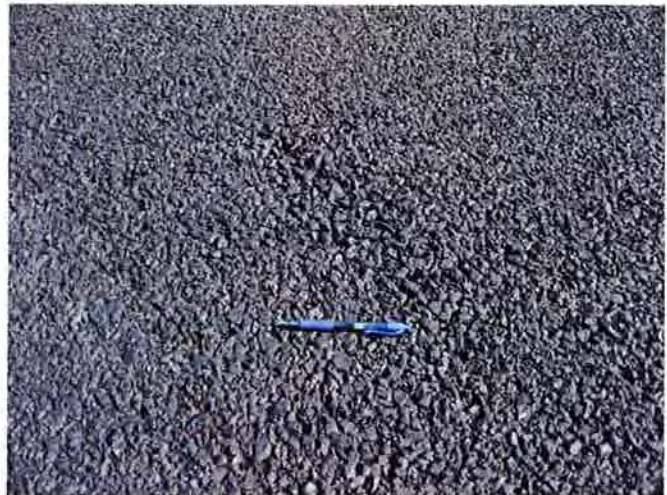
A-2, Surface detail with raveling
