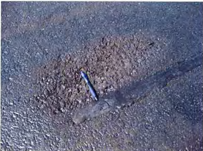
A-2, Surface detail with crack and raveling
