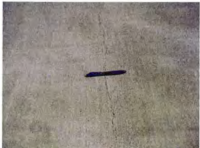
A-4, Surface detail with crack
