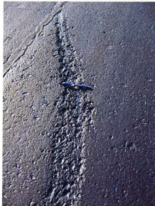
T-2, Surface detail with crack and raveling
