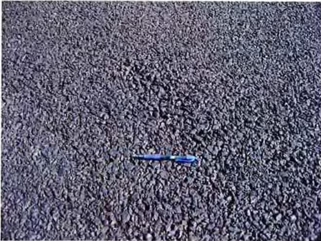
A-1, Surface detail with raveling
