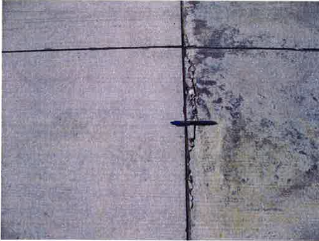
A-4, Surface detail with spalling
