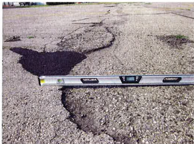
A-3A, Surface detail with depression and raveling
