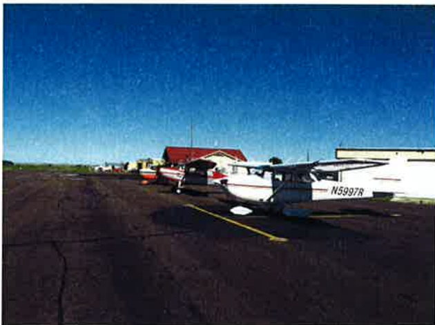
A-5, Overview with cracks and depressions
