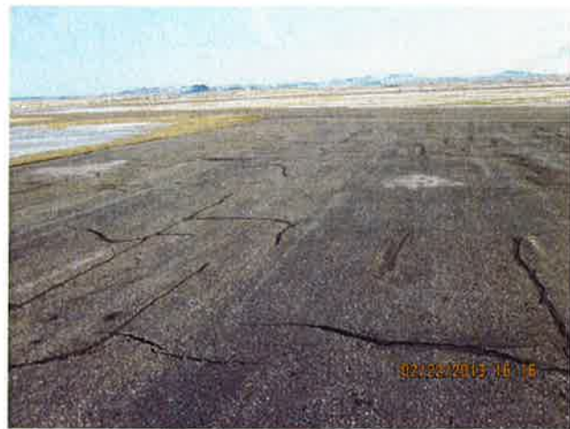
A-3, Overview with cracks
