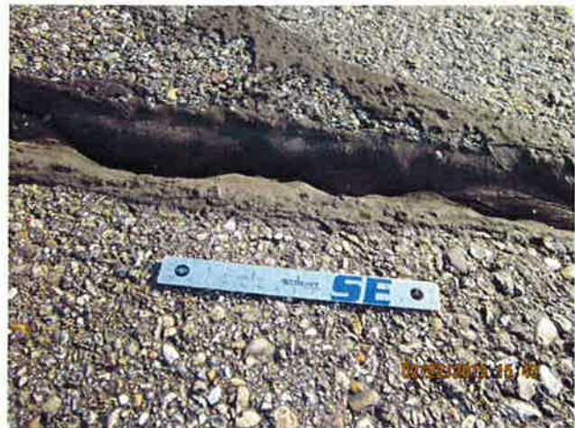
T-3, Surface detail with crack
