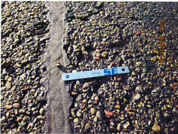
A-5, Surface detail with crack
