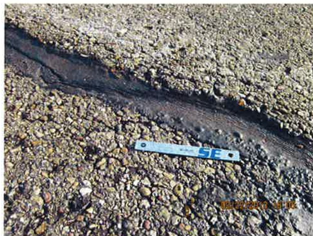
A-5, Surface detail with crack
