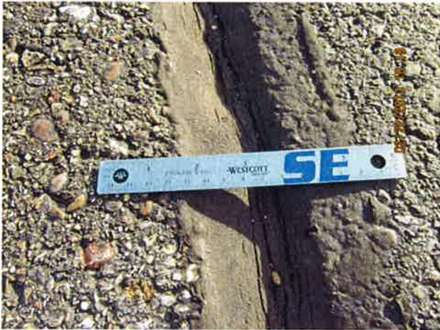
T-5, Surface detail with crack
