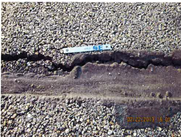
R-5, Surface detail with crack
