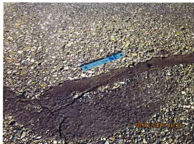
A-3, Surface detail with crack
