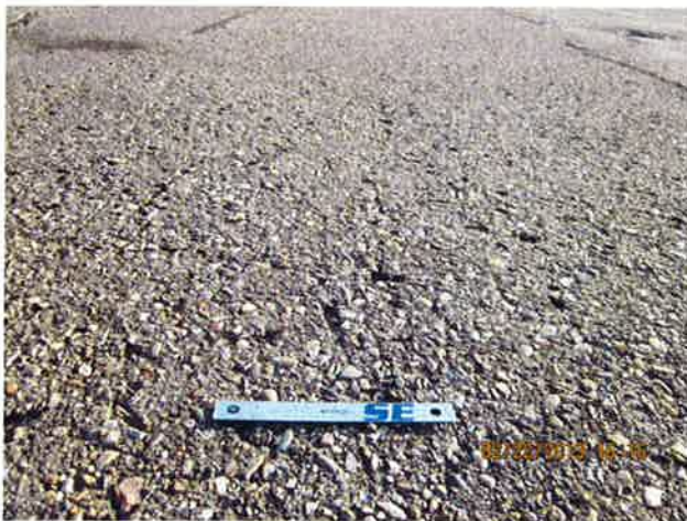
A-3, Surface detail with raveling
