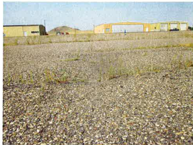
A-4, Surface detail with cracks and depressions
