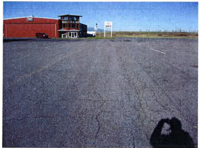
A-2, Overview with cracking
