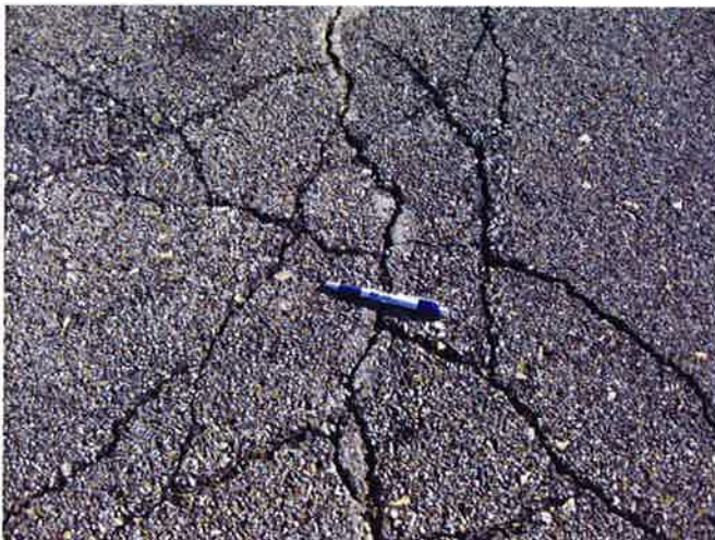
T-3 , Surface detail with cracking
