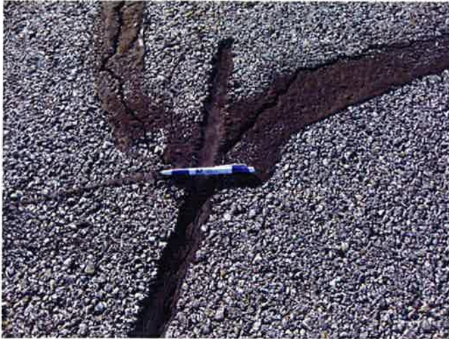
R-2 , Surface detail with crack
