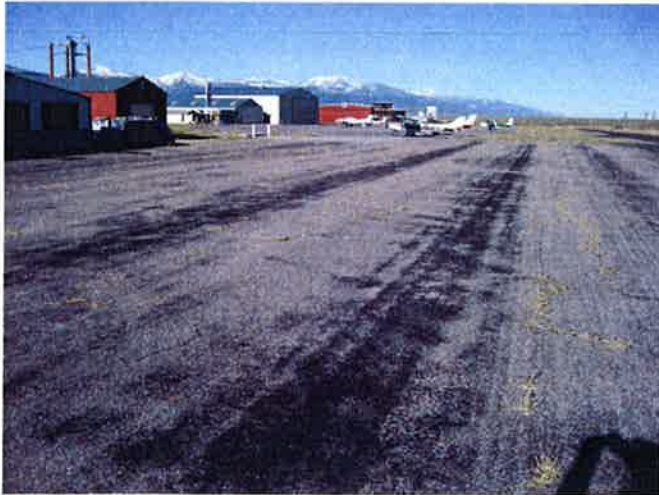
A-1, Overview with bleeding
