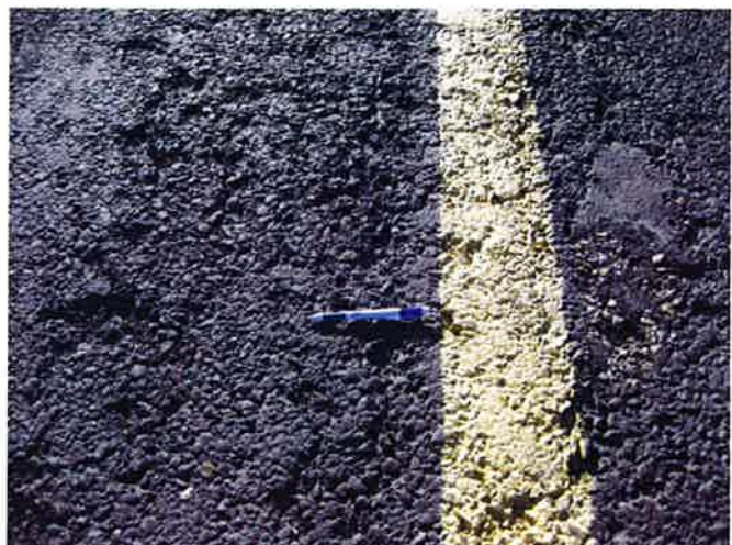
T-3 , Surface detail with raveling
