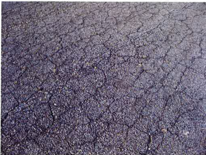
A-2, Surface detail with cracking
