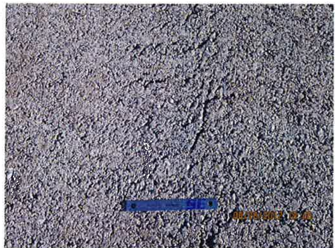
R-11, Surface detail with cracking
