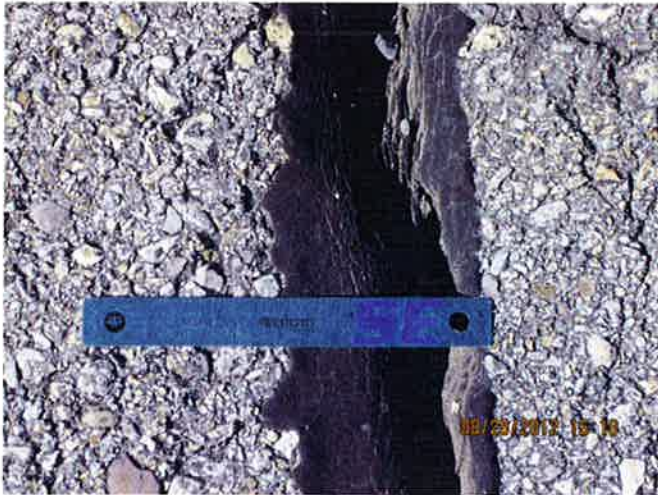
A-1, Surface detail with crack
