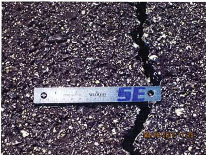
A-2, Surface detail with crack
