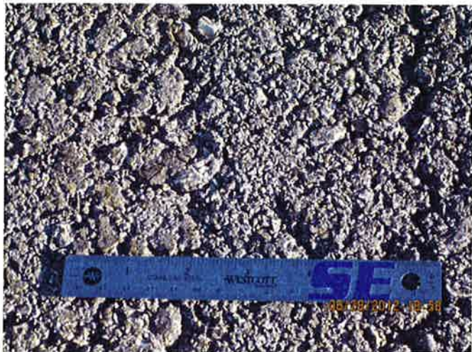
R-11, Surface detail with weathering and crack
