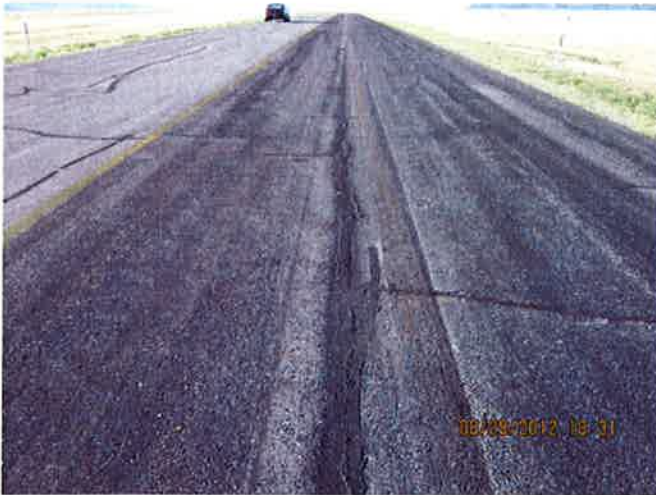
T-2, Overview with cracks and depression
