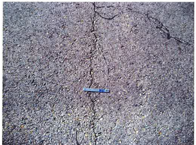
A-1, Surface detail with cracking
