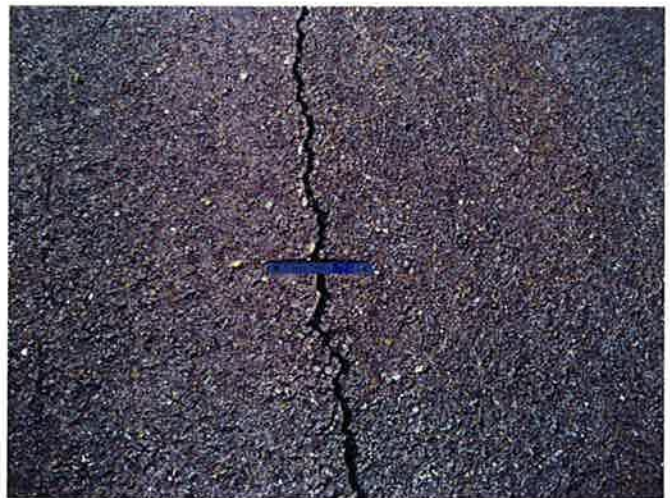
R-3 , Surface detail medium severity crack
