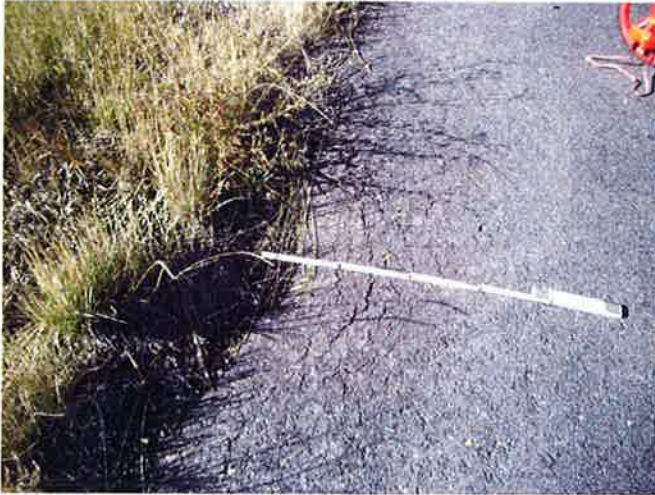
T-4, Surface detail depression with alligator cracking
