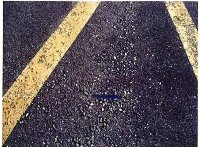
T-4, Surface detail raveling
