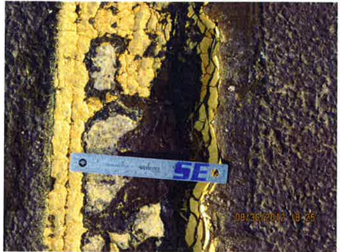
A-1, Surface detail with crack
