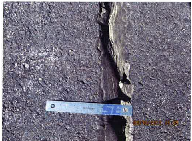
R-1, Surface detail with crack
