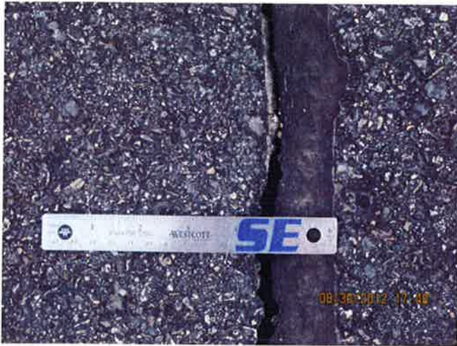
T-2, Surface detail with crack
