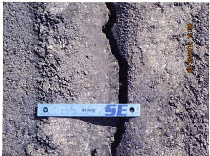
T-1, Surface detail with crack
