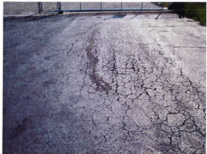
A-1A, Surface detail with cracking
