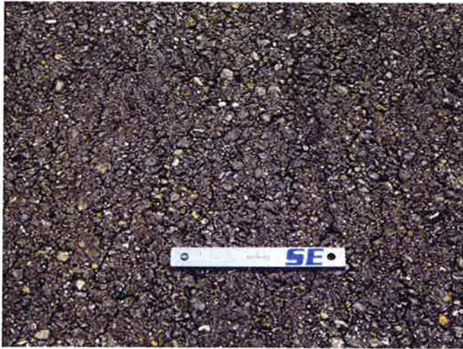
A-1B , Surface detail with cracking
