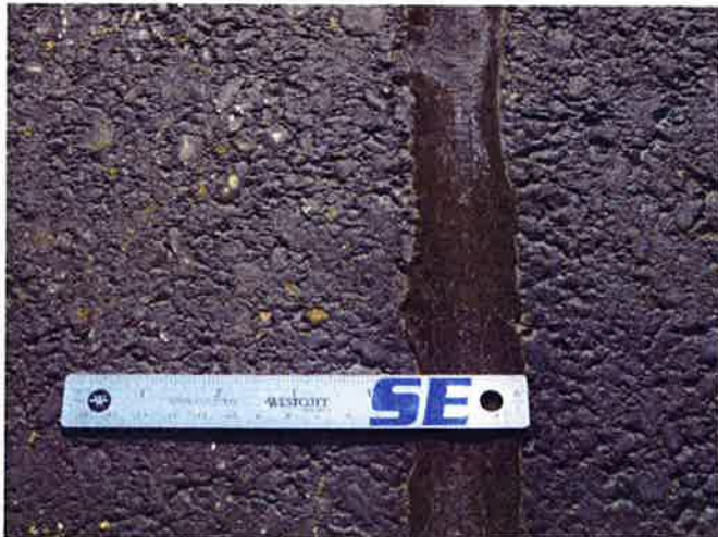
A-1A, Surface detail with crack
