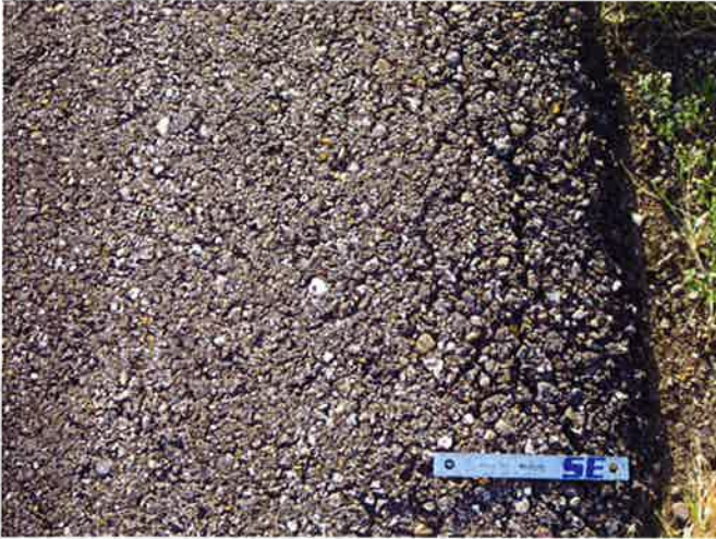
T-1, Surface detail with cracking
