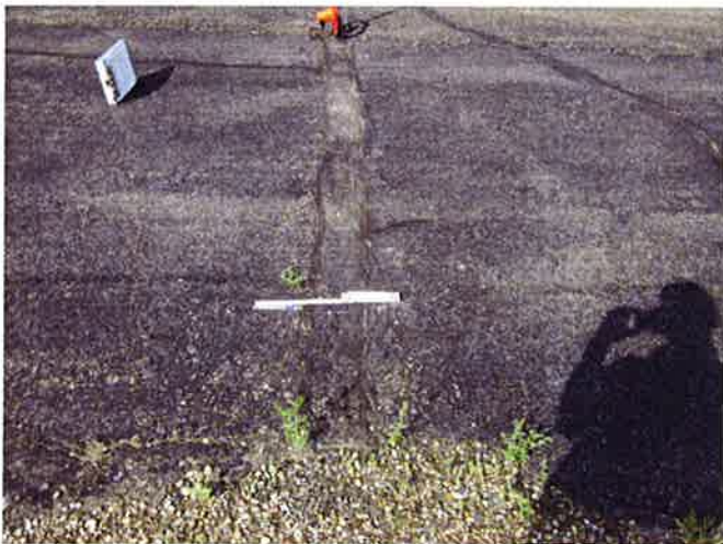
T-1 , Surface detail with patching (50)
