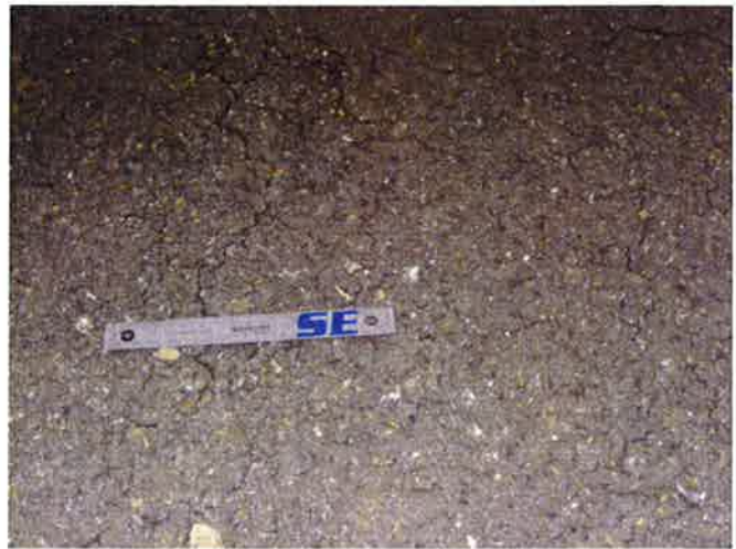
R-11 Surface detail with cracks
