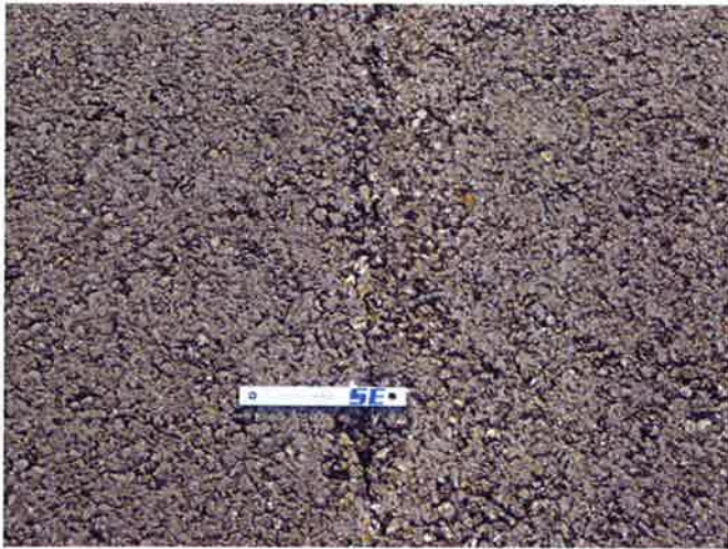
R-11 , Surface detail with crack
