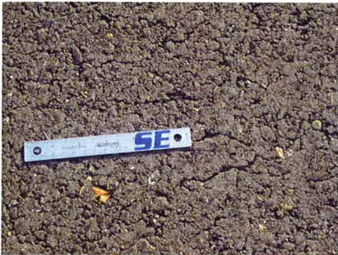
A-2, Surface detail with cracks
