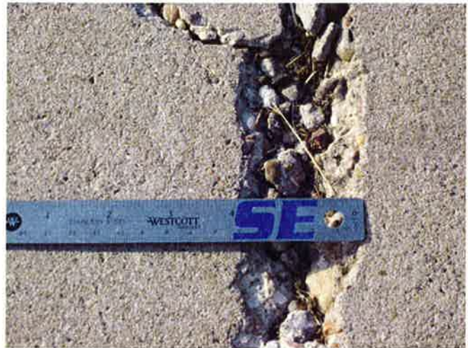
A-1, Surface detail with crack
