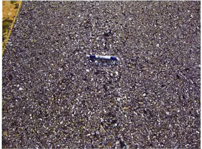
T-5, Surface detail with raveling
