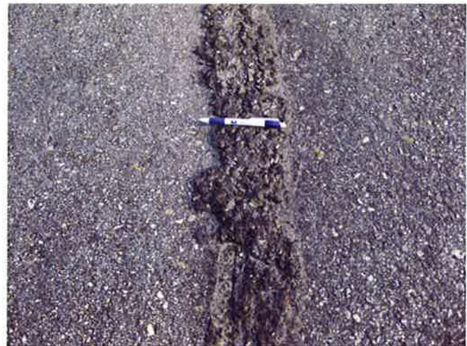
T-4 , Surface detail with crack and patch
