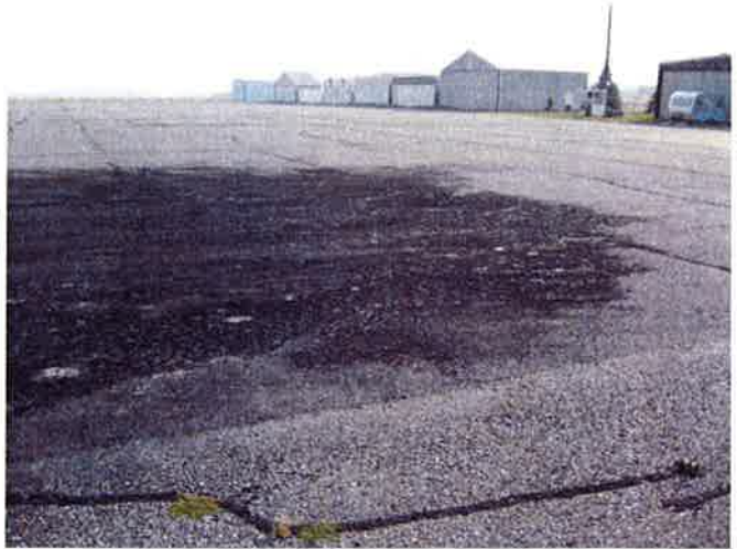
A-2, Overview with crack and raveling
