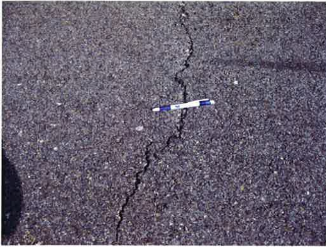
R-1 , Surface detail with crack
