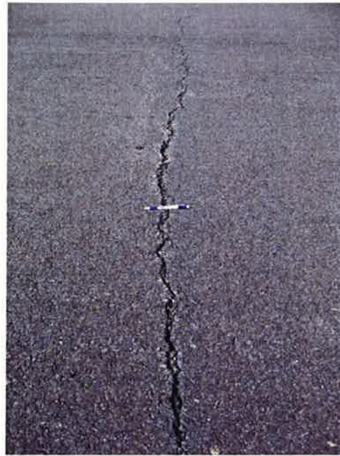
R-1 , Surface detail with cracking
