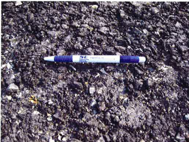
A-2, Surface detail with raveling
