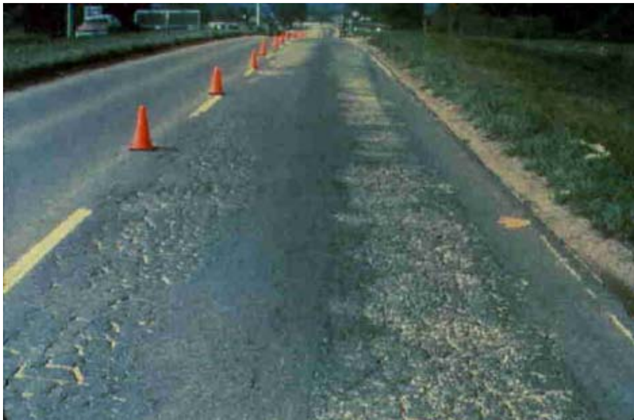
Figure 9-1 Deteriorated Asphalt Pavement and Candidate for Recycling
