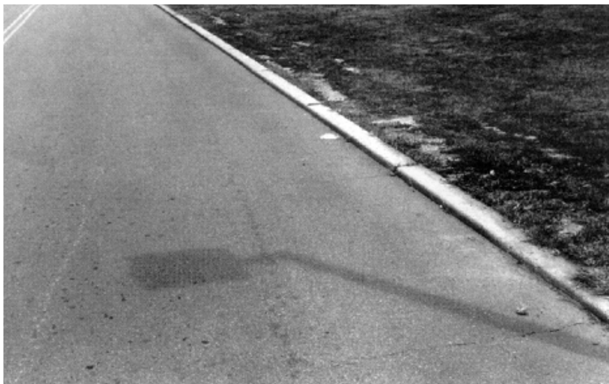
Figure 9-2 Loss of Curb Height/Reveal and Drainage Capacity
