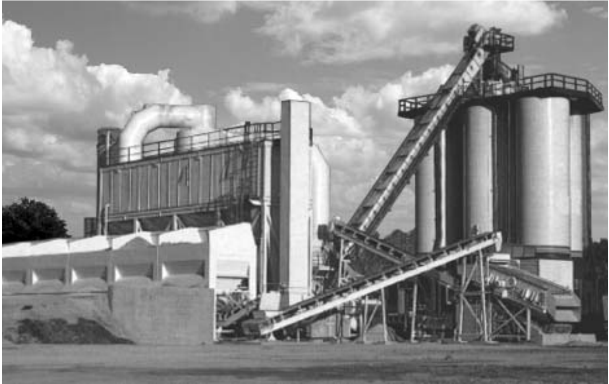
Figure 1-5: Asphalt batch plant with RAP infeed for hot recycling
