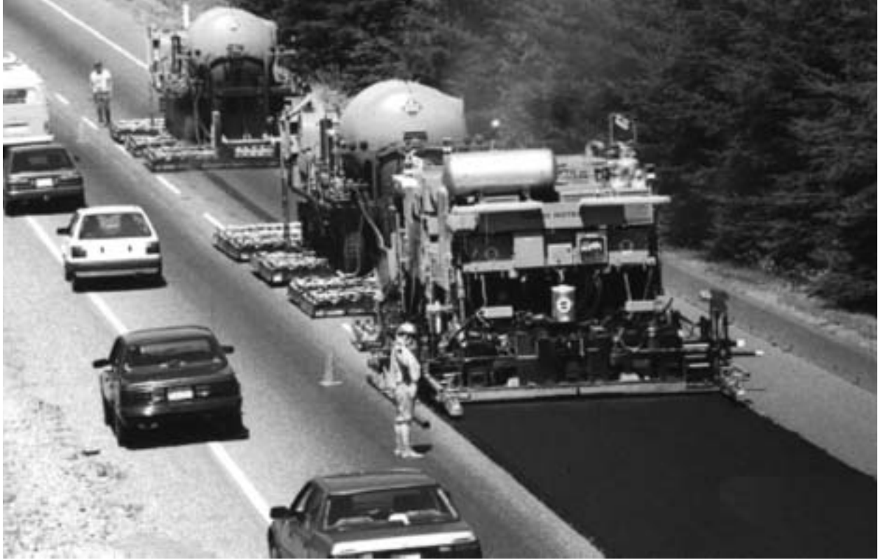
Figure 1-11: Single stage Remixing train
