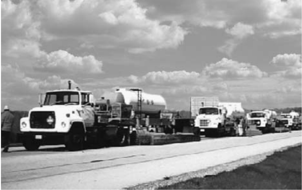
Figure 6-1: Surface Recycling preheaters
