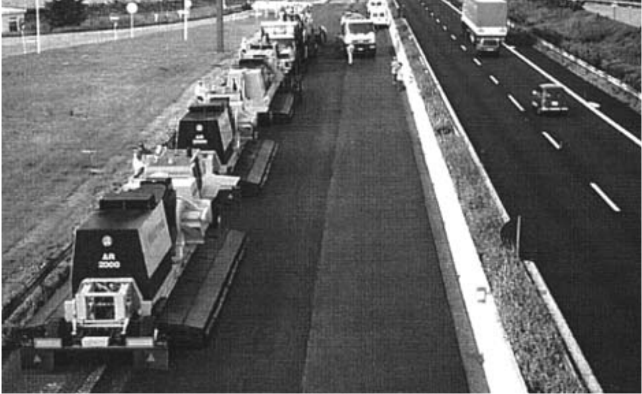
Figure 6-11: Single stage Remixing train
