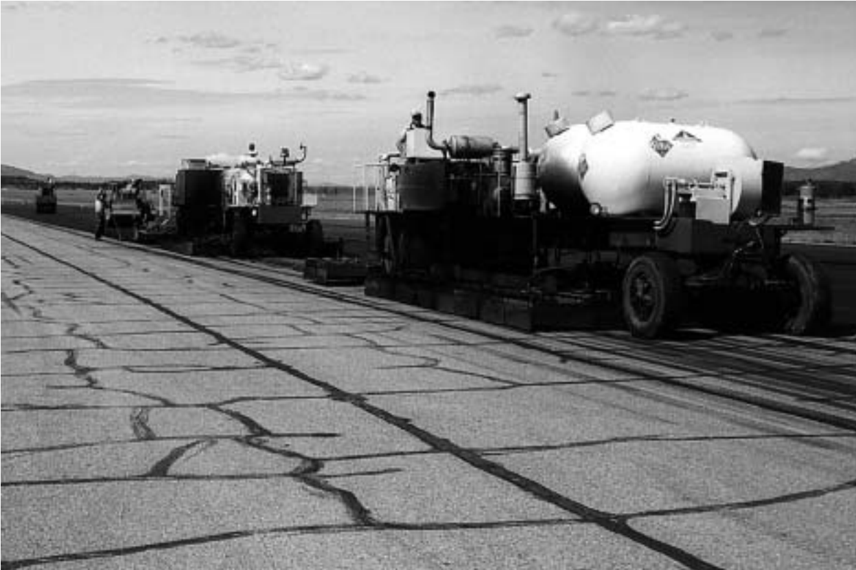
Figure 1-7: Surface Recycling heating units
