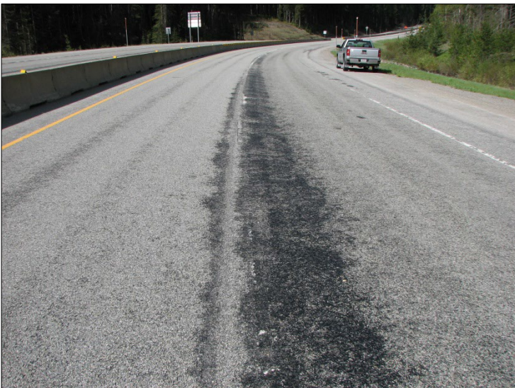
← Additional image of surface flushing on the FSCS section.
