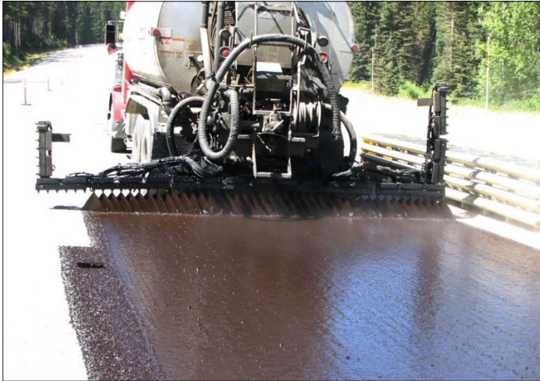
← Typical application of CRS-2P emulsion (50/50 diluted with water), by asphalt distributor truck. Dilution blend was done at plant.
