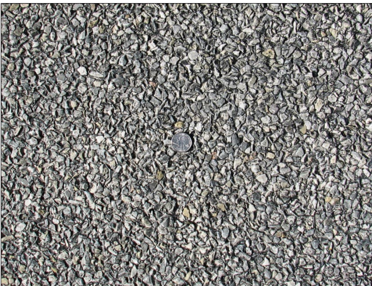
← Close-up of intact FSCS surface texture.
