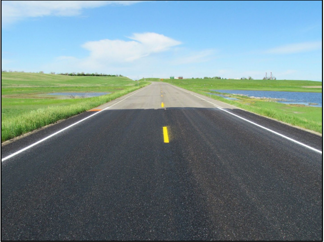
↑ End of CSS-1H fog seal over CRS-2p project section; west end, view west at approximate RP 355.
