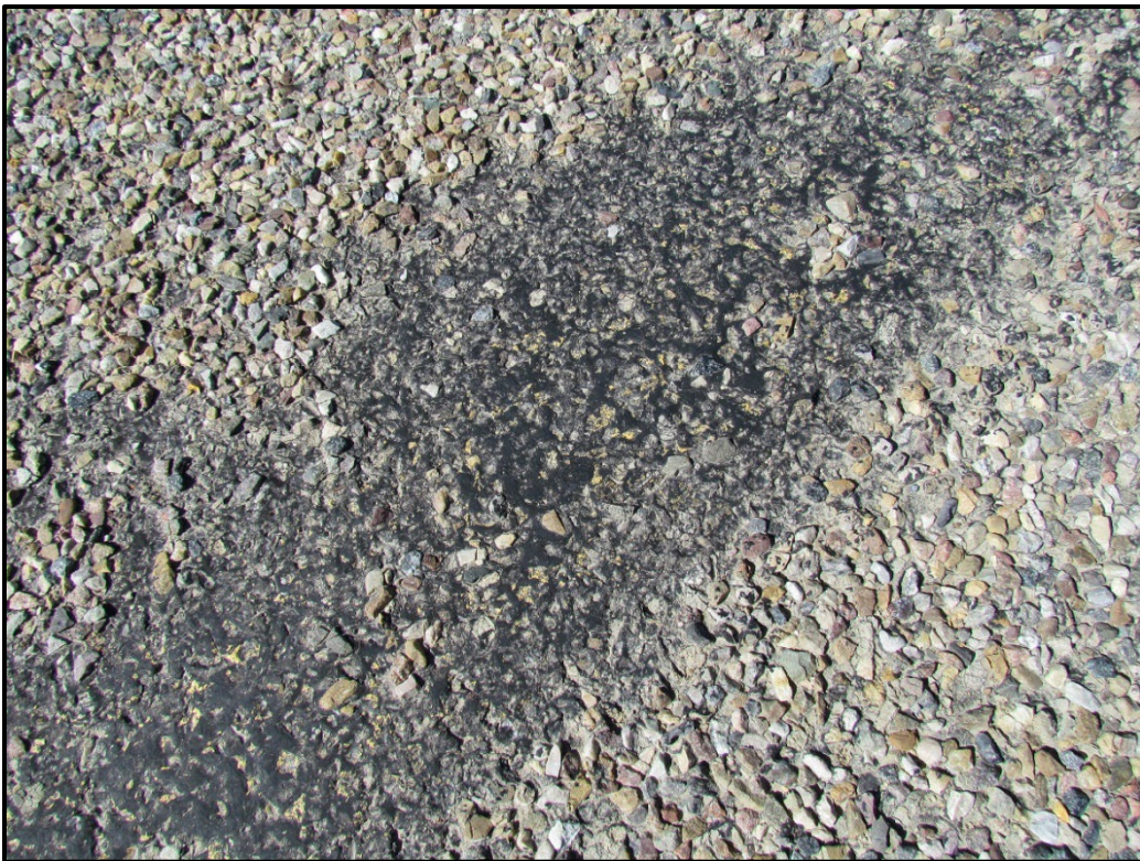
↑ Close-up of centerline chip loss.
