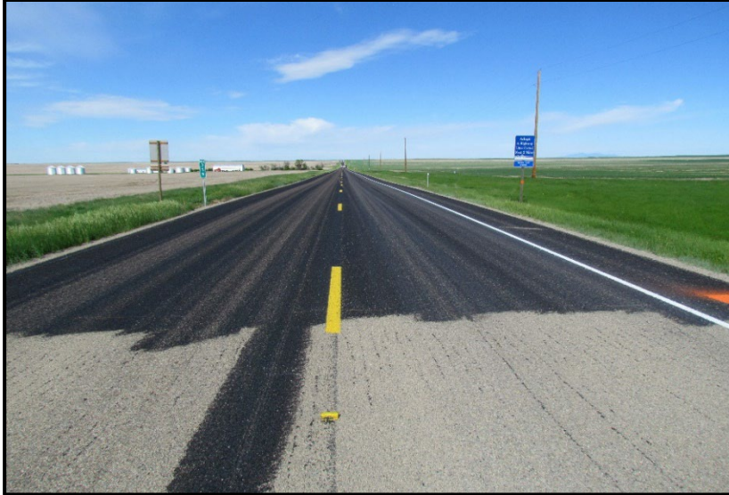
← Begin of CSS-1H fog application on CRS-2p section at RF 359 view west.
