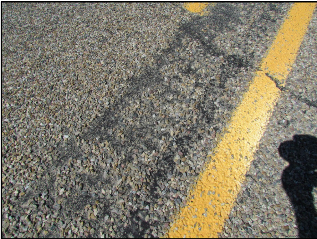
↑ Close-up of centerline chip loss.
