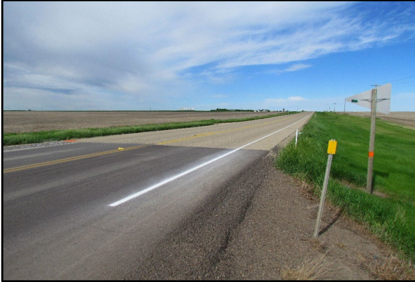
← Completion CRS-2p without fog seal section after sweeping. View is at RP 363, view west.
