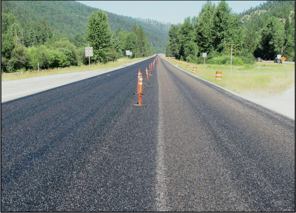
↑ Both lanes with completed FSCS application. Driving lane has active traffic while passing lane is allowed to completely cure.
