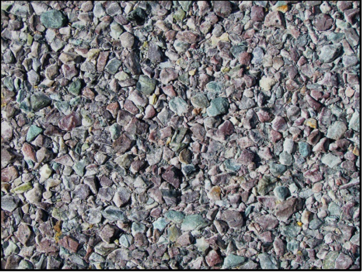
← Close-up of chip seal using MDT Type III aggregate with CHFRS-2p emulsion.
